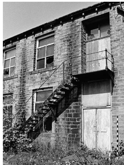
Photo 3. Loading doors and landing
