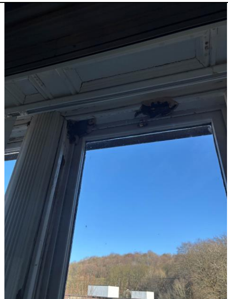
Photo 3 – Area under box gutter and window decay.
