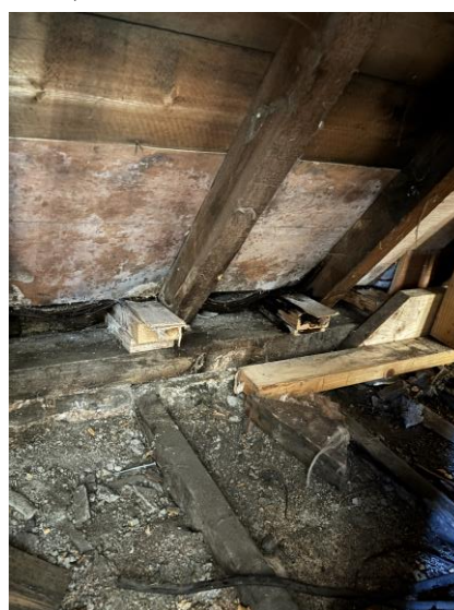
Photo 2 – Area of water ingress from box gutter
