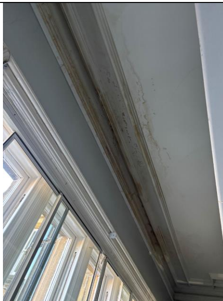
Photo 4 – Area under box gutter showing dry rot extent
