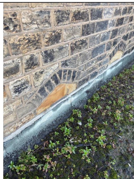
Photo 6– Stable block upstand deterioration.
