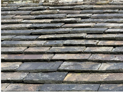
Figure 3 – Existing natural stone slate roofing materials to be retained and reinstated around the proposed opening.
