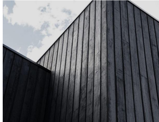
Charred timber cladding to Plot 4
