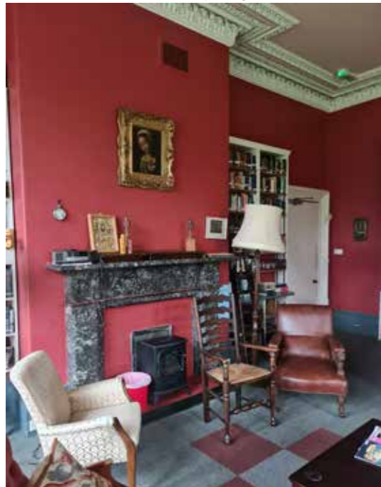
Low quality floor finishes (Main House)
