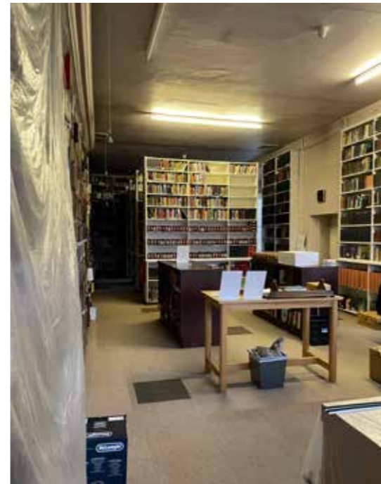
Library Wing (Main House, first floor) - poorly maintained
