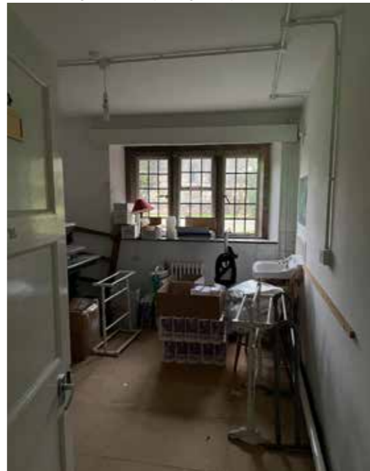
Neglected and cluttered spaces throughout
