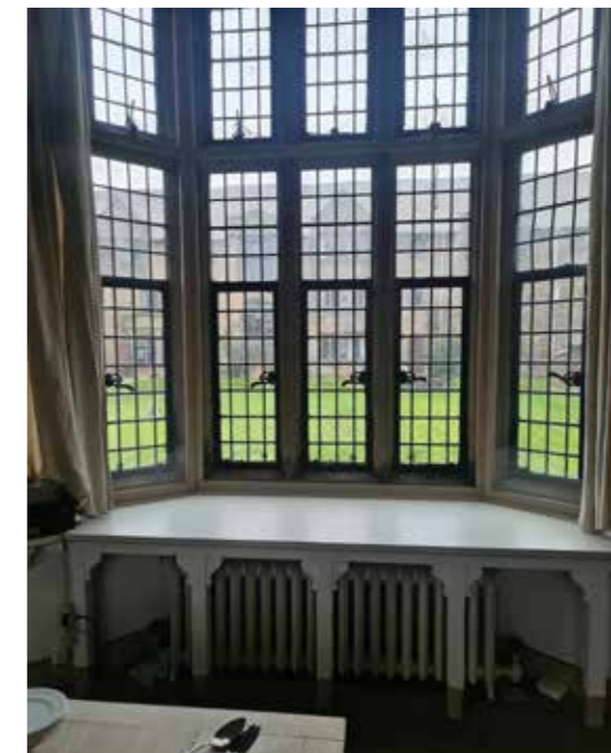
Leaded lights requiring maintenance, lose services and jointery restricting warm air flow from radiator below.
