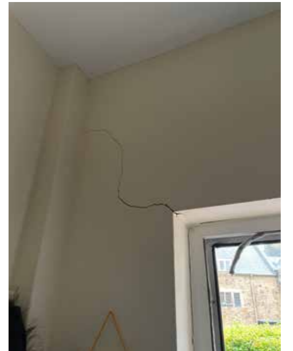
Visible cracking internally
