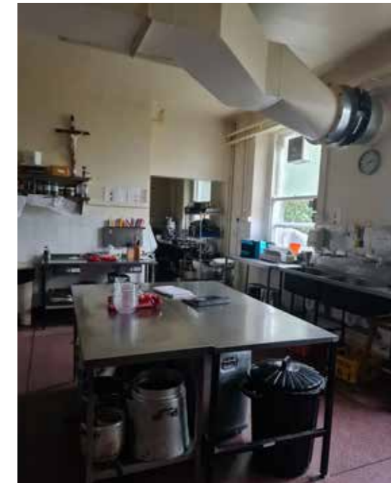
Kitchen - Intrusive services and negative impact on plan.
