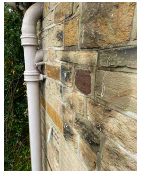
Saturated areas of stonework externally
