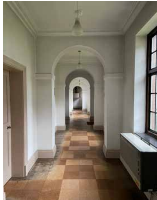
Floor damage to Library Wing with platform lift in view
