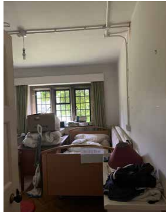
Infirmary Room (East Wing) - poorly planned / maintained
