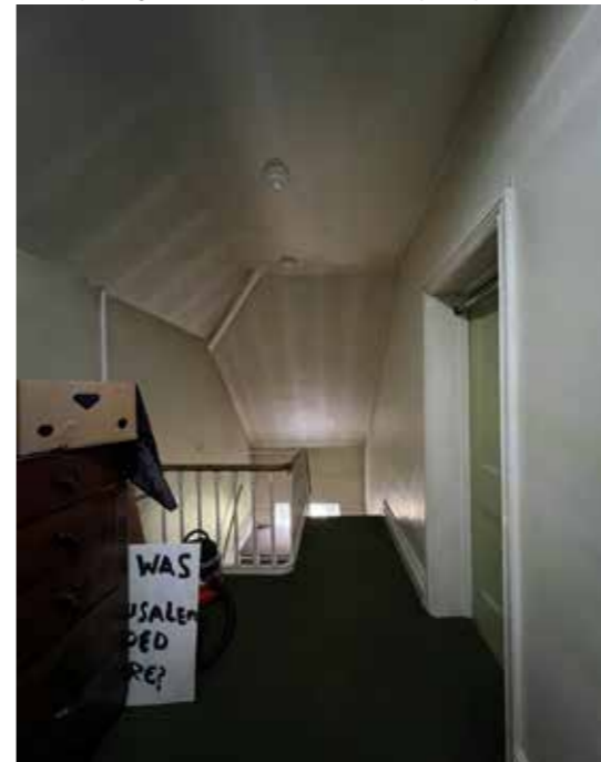
Attic - lacking maintenance / adequate heat or vent
