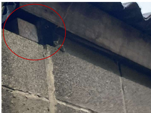
Photo 13: Gap in the eave on the northeastern aspect.
