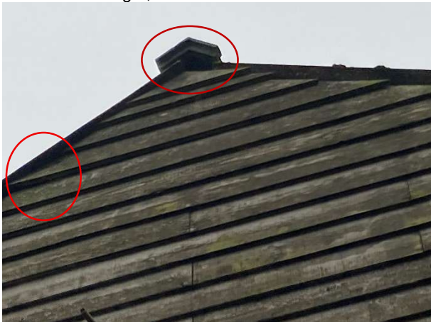
Photo 11: Gap under ridge tile and cladding on the northern aspect of Building 1.
