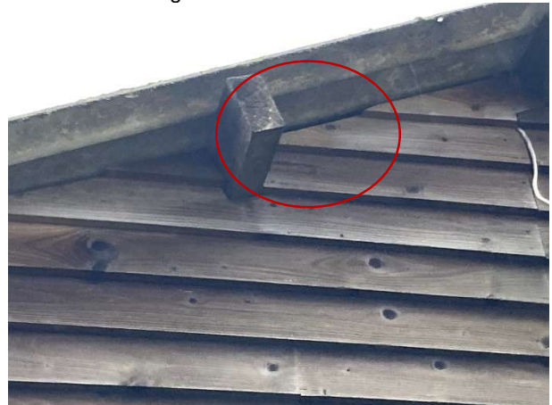
Photo 12: Gap in the Eave on the southern aspect of Building 1.
