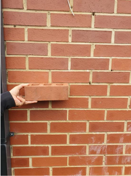
Above: Proposed red brick, these are standard red sand faced that match neighbouring properties, to be used on rear elevation.
