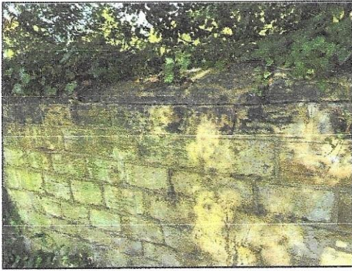
Photo 1: Lateral Movement of Wall
