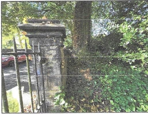
Photo 3: Tree Trunk Impacting Wall
