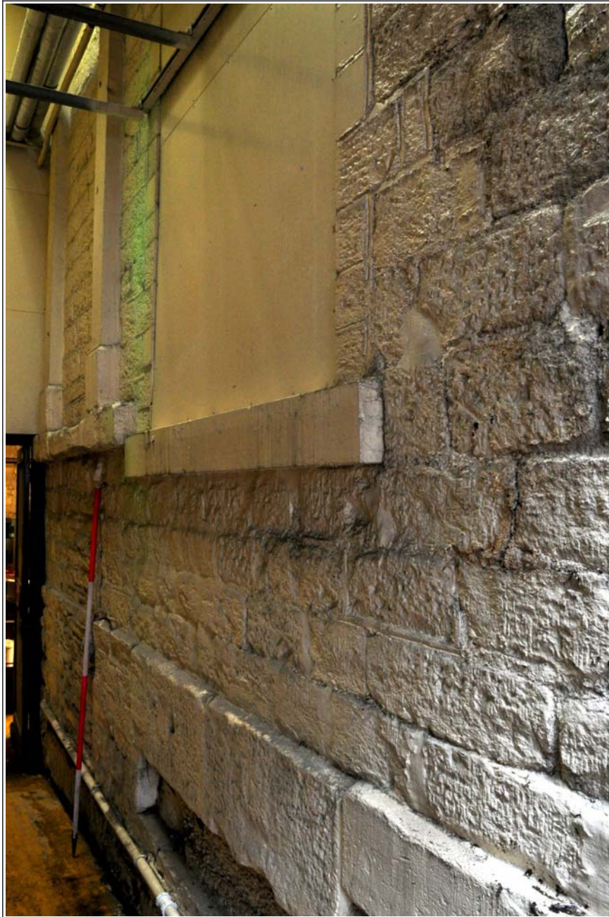
04: Openings at ground floor level, north elevation (doorway and later window), looking east
