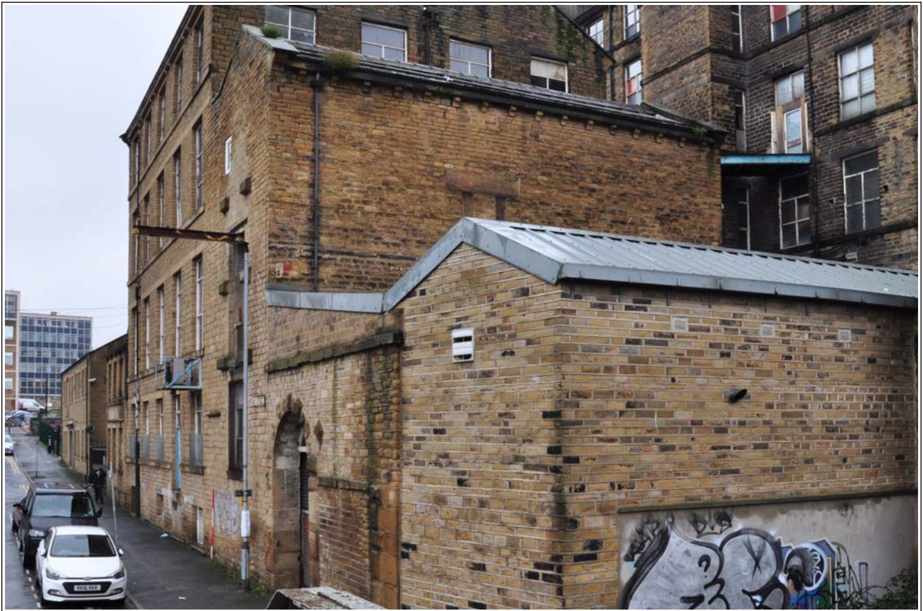
01: General view of former engine house from the south-east; former boiler house in foreground
