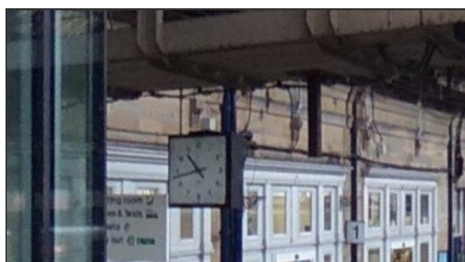
Insert 4-35 - Images depicting the existing analogue platform clocks, to be removed to prevent damage and later reinstated either at Huddersfield Station or another appropriate Network Rail site.
