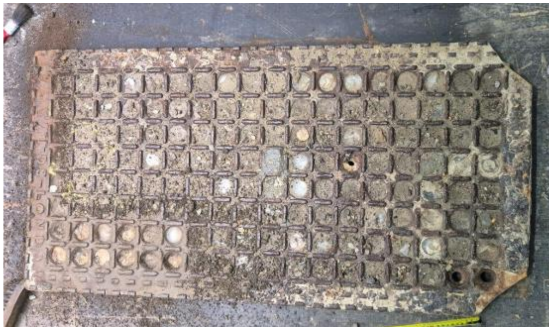
Insert 4-31 – Condition of the pavement light once removed from platform, showing damage at the corners and the glass, see Appendix C.6 for more details.
