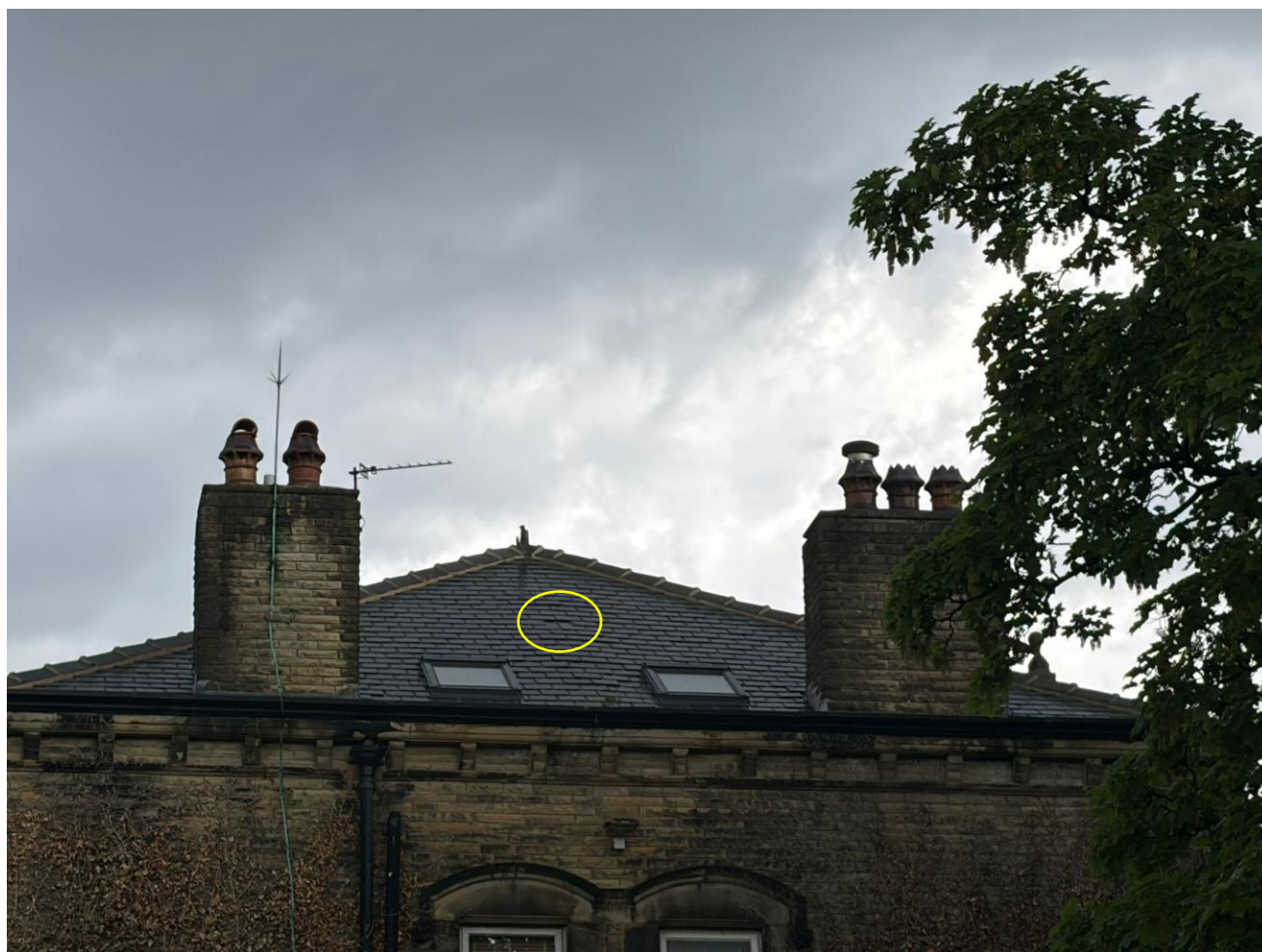
Figure 3 – Missing tiles present on the southern aspect of the property B1
