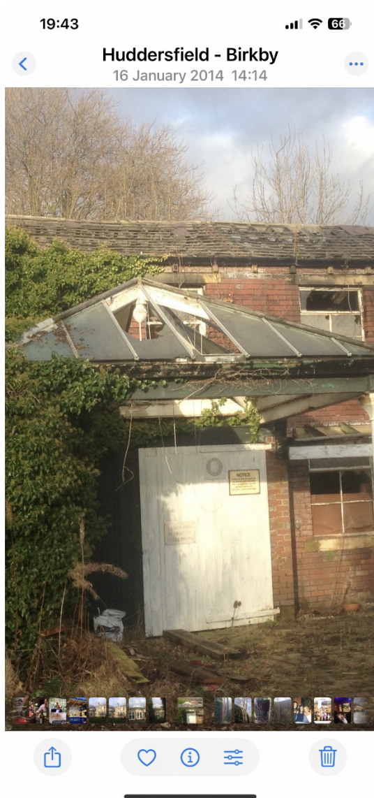
Photo shows the existing building with the roof slates removed and the start of glazing removal and vegetation dated 16 of January 2014.
