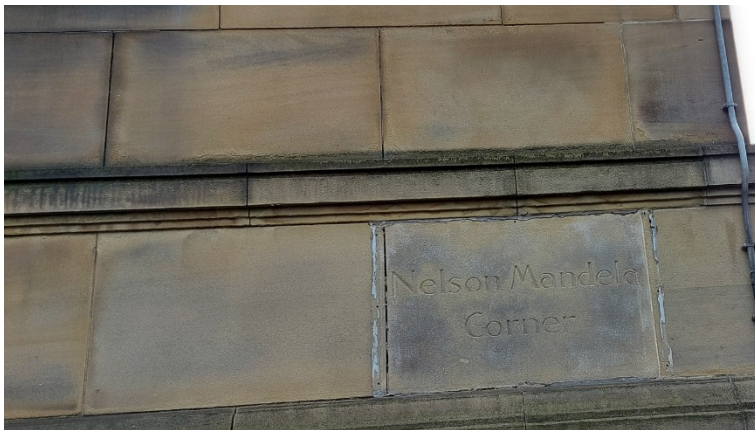
Plate 11: Example of the open mortar joints to the facades.
