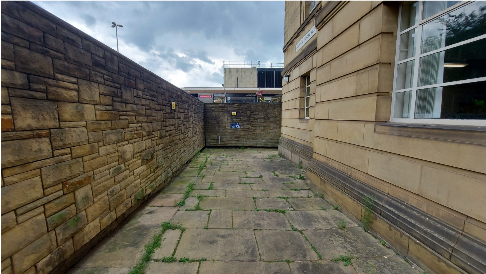
Plate 12: The area of the proposed amenity space and new structures, showing the modern retaining wall as existing.
