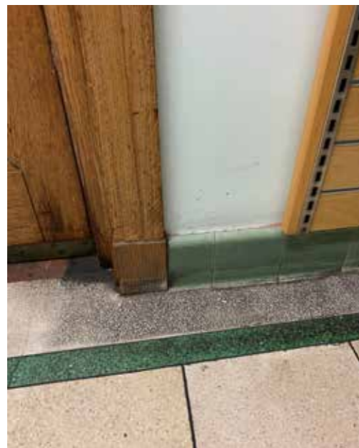
4.8.16 - Architrave to Boys WC (Rm.23)
