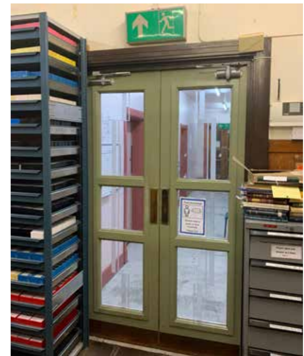
4.6.15 - Doors in Reference Archive (Rm.66)
