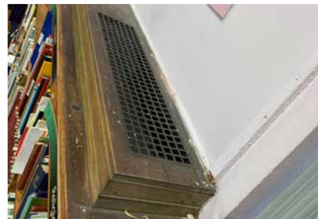
4.6.11 - Ventilation in Local History Library (Rm.68)
