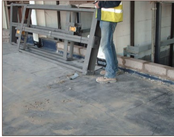
Figure A4.50 Large/heavy/sharp objects being moved over unprotected gas membrane (courtesy Card Geotechnics Limited)
