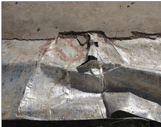
Figure A4.54 Gas membrane damage/tearing at edge of ground floor slab screed layer where it was left exposed to elements for period of time (courtesy NHBC)
