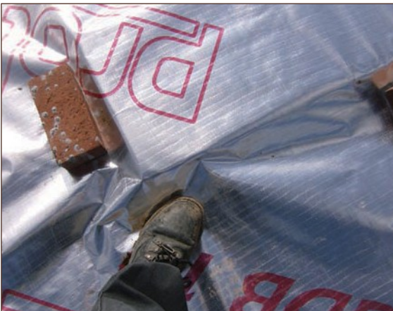
Figure A4.71 No corner detailing leading to stress point on gas membrane (courtesy Smith Grant)
