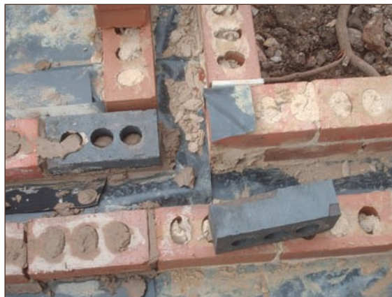
Figure A4.66 Follow-on trades proceeded work before gas membrane joints sealed (courtesy Card Geotechnics Limited)
