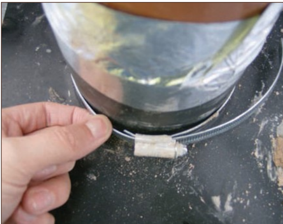
Figure A4.75 Jubilee clip on service entry insufficiently tightened so joint is uncompressed (courtesy Smith Grant)
