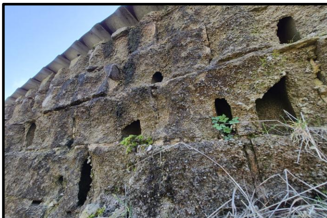
Photograph 7. Example of weathered blocks on northern aspect of Building 1
