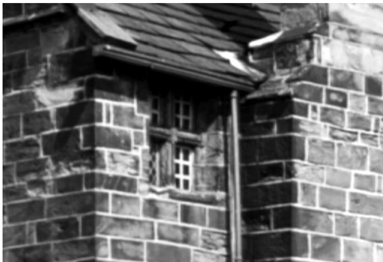
Photo c. 1900. Cast iron gutters and pipes set proud of the wall without cast iron swan necks.
