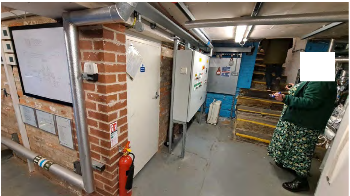
Photo 89: Modern boiler equipment in cellars
