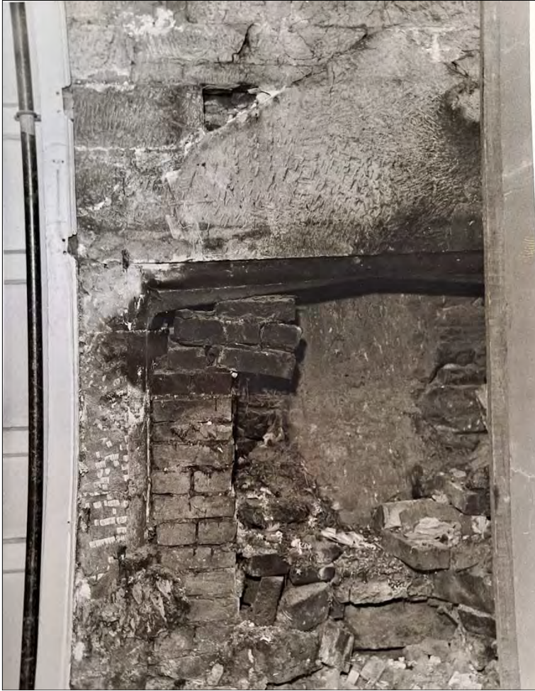
Figure 18: Fireplace in room now used for toilets
