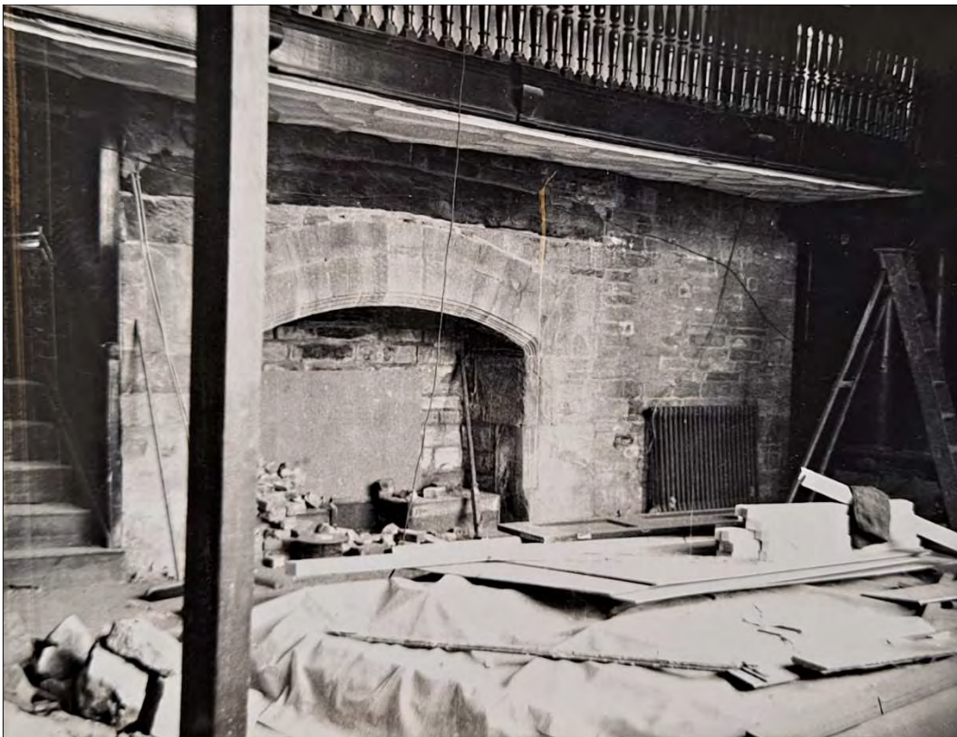
Figure 15: The fireplace in the Great Hall after removal of 19th century additions
