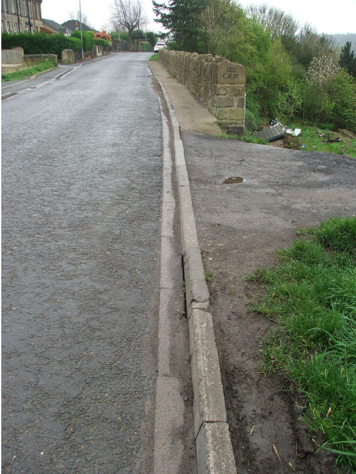
Kerb line across site access showing displaced transition kerb and cracked full kerb.
