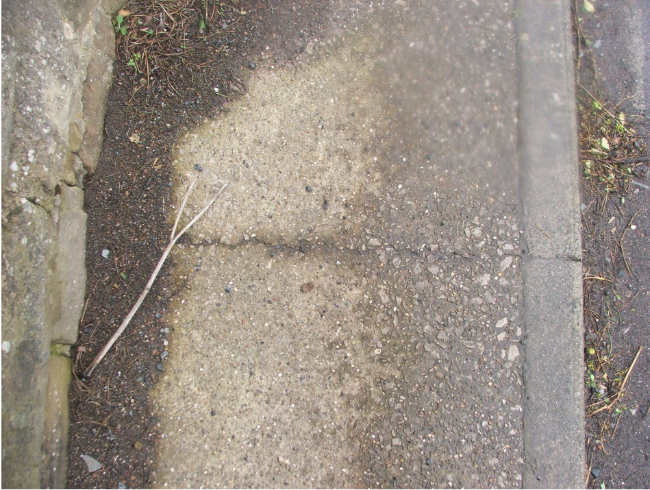
Typical shrinkage crack concrete verge.
