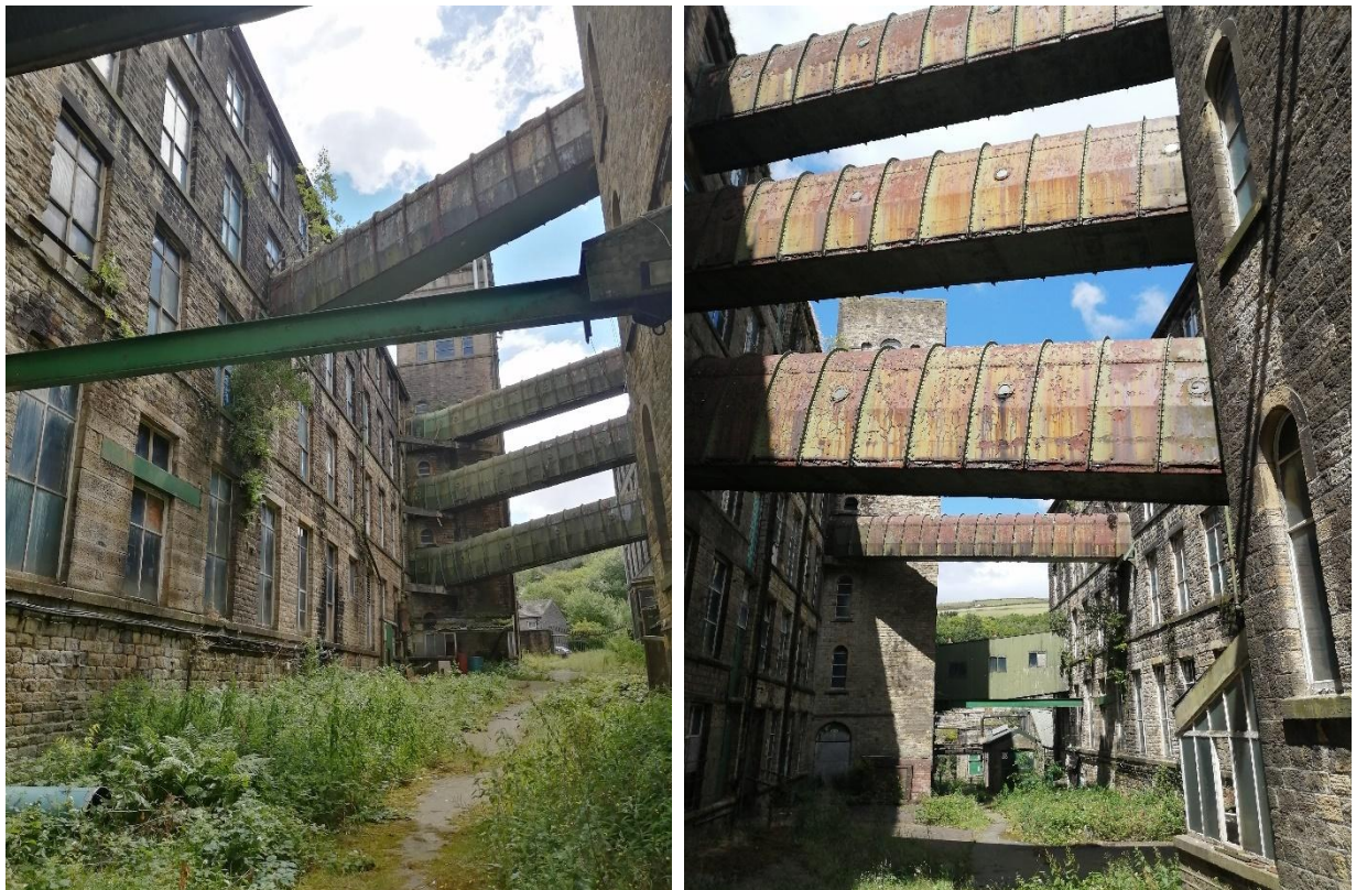
Figure 12 The space between the two multi-storey blocks, A and B, is narrow and its drama is enhanced by the high-level tunnel connections.
