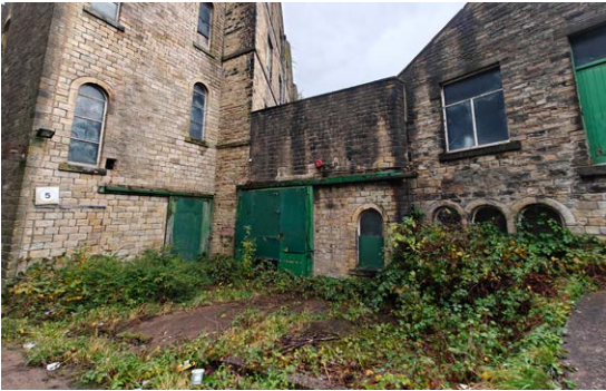
The green colour of doors and other features against the buff Yorkshire brick is a distinctive characteristic of the site
