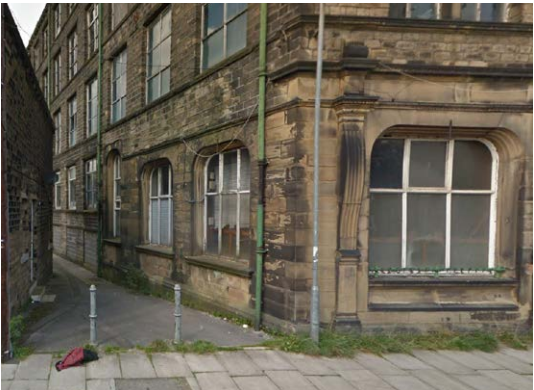
A view along the west side of the Wages Office showing the link through to Derby Terrace
