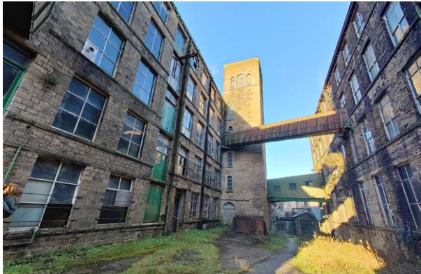
Between the east and west mill buildings showing the elevated bridge links
