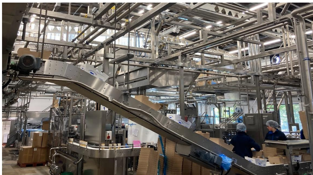
Equipment in the existing cottage cheese department at Longley farm
