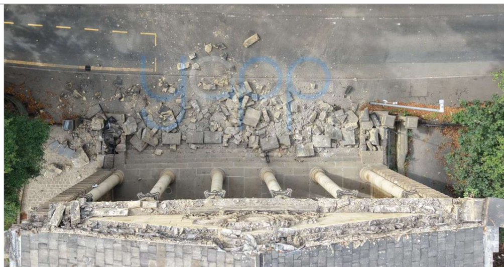
Photo 3: Drone footage taken directly after the collapse (taken from 'Yapp App')
