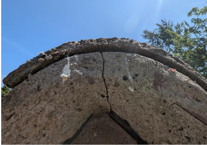
Plate 3.2. Slightly lifted ridge tile.
