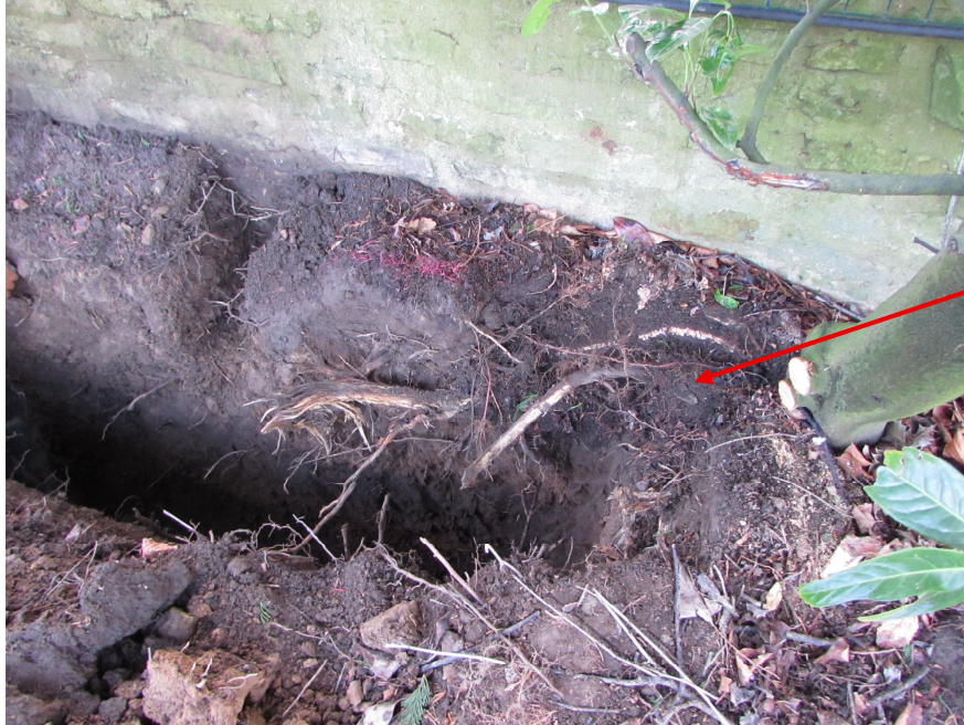
Photo 5 – Trial Pit 2 Showing the roots going to the Laurel.
