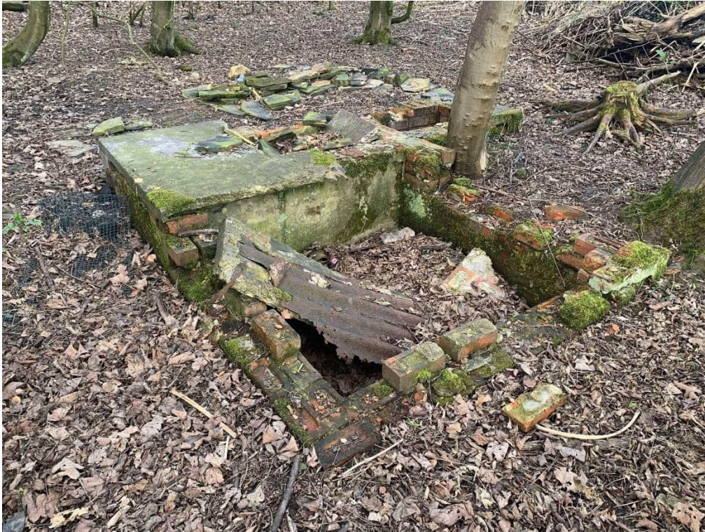
View of the demolished structure to the central south of the western side of the site, facing east.
