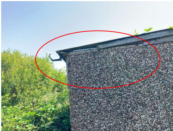
Photo 13: Missing barge board on the western aspect of the most eastern flat roofed extension.
