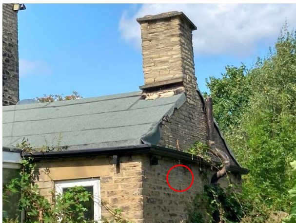
Photo 9: Air vent on the eastern aspect of extension.
