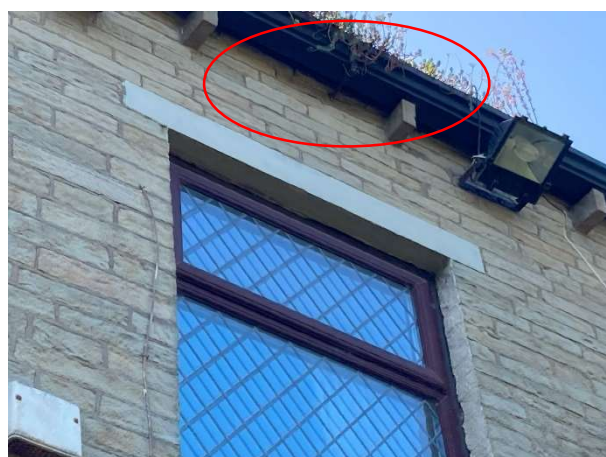
Photo 6: Gap in the eave in the northern aspect of the building.
