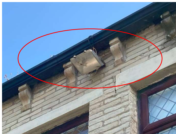
Photo 10: Gap in the eaves on the southern aspect of the building.
