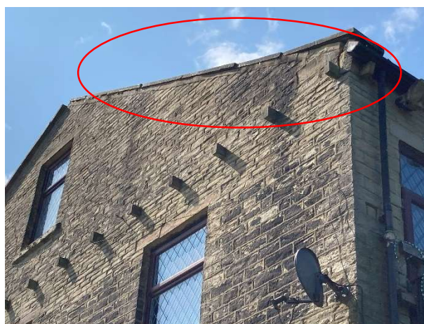
Photo 8: Gap in the eaves on the eastern aspect of the building.
