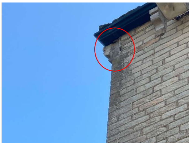
Photo 11: Missing mortar on the southern aspect of the building.
