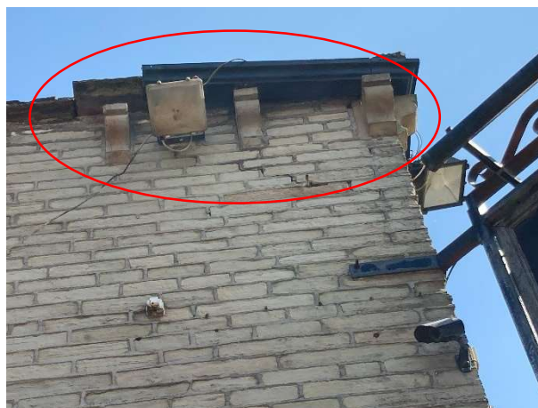
Photo 12: Gap in the eaves and missing mortar on the western aspect of the building.
