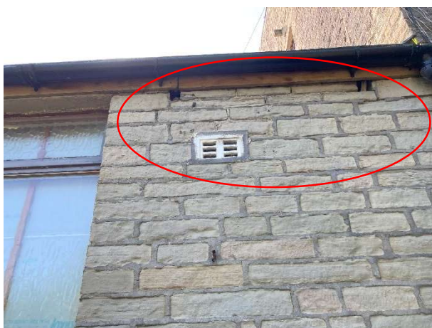
Photo 7: Missing bricks and air vent on the northern aspect of the extension.
