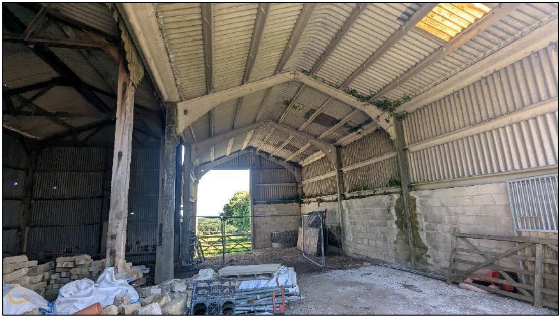
Plate 6. Gaps between concrete blocks in south elevation wall
