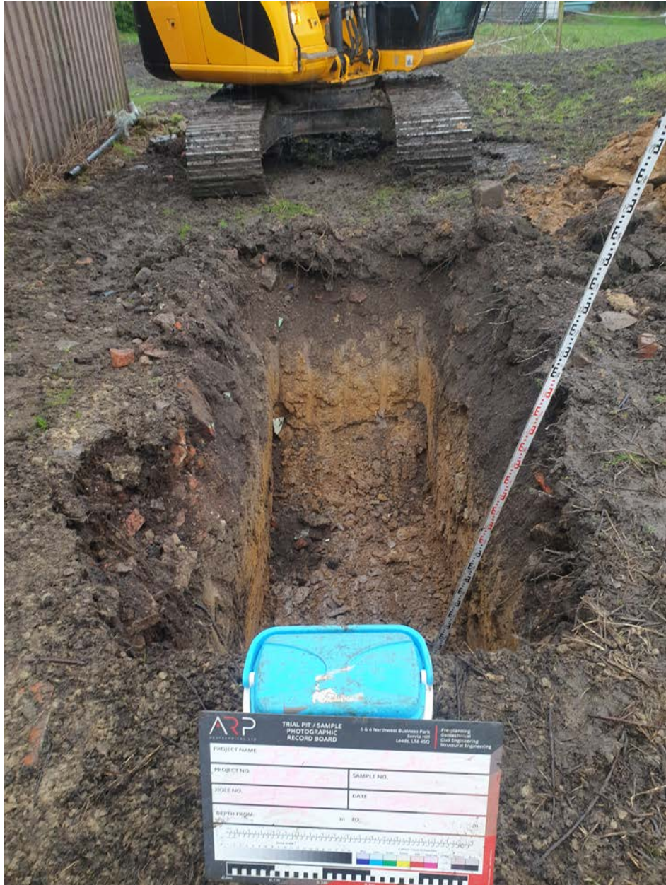
Photograph 3: Looking west, from north of existing building, across TP01, excavated to rockhead.
