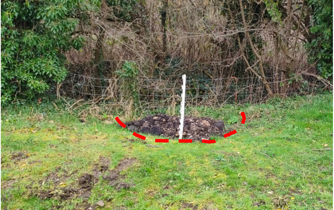
Photograph 1: Looking West, at the western boundary, at depression highlighted.
