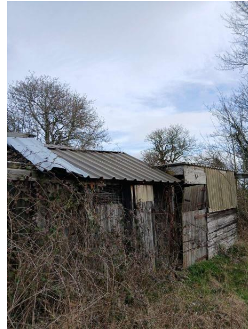
Photo 2: Building to the north of site (B1), subject to degradation.
