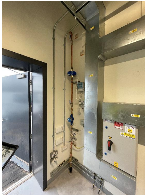
Fig 11: Main Water Meter in the Utility Room.
