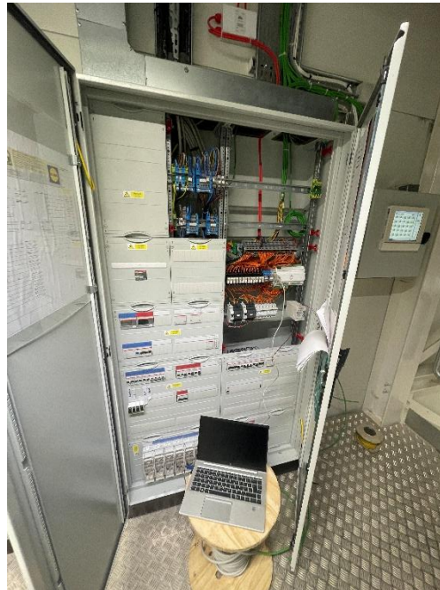
Fig 9: BEMS Control Panel.
