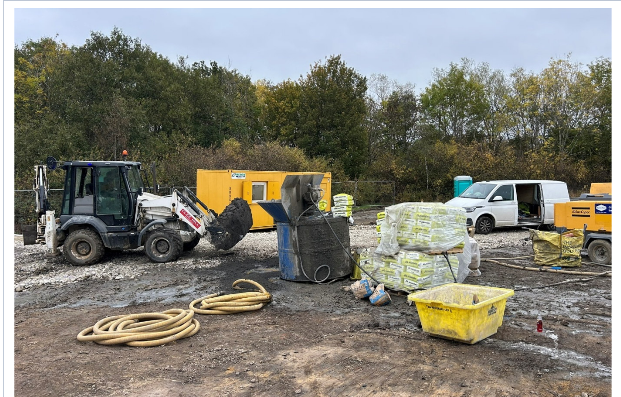
Photograph 3 – Photograph of grout mixing equipment.
