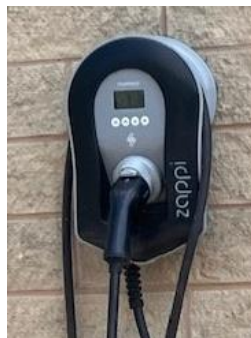
Example of EV charger
