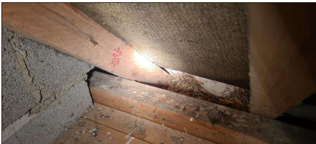
Plate 16. Bird's nest in the soffit of the garage
