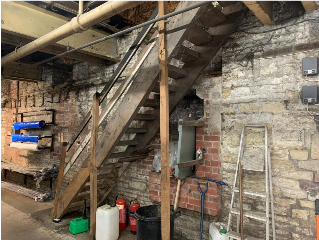
Figure 4 – Photograph taken inside the Lower Ground Floor showing the existing staircase, the only access to the Lower Ground Floor at present from the upper floors
