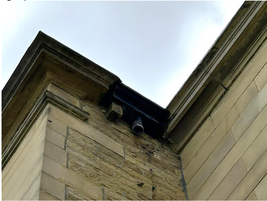
Photo G: Small section of existing (probably cast iron) gutter to Acre House adjacent to front elevation. New aluminium gutter of similar ogee profile to be fitted & continued
