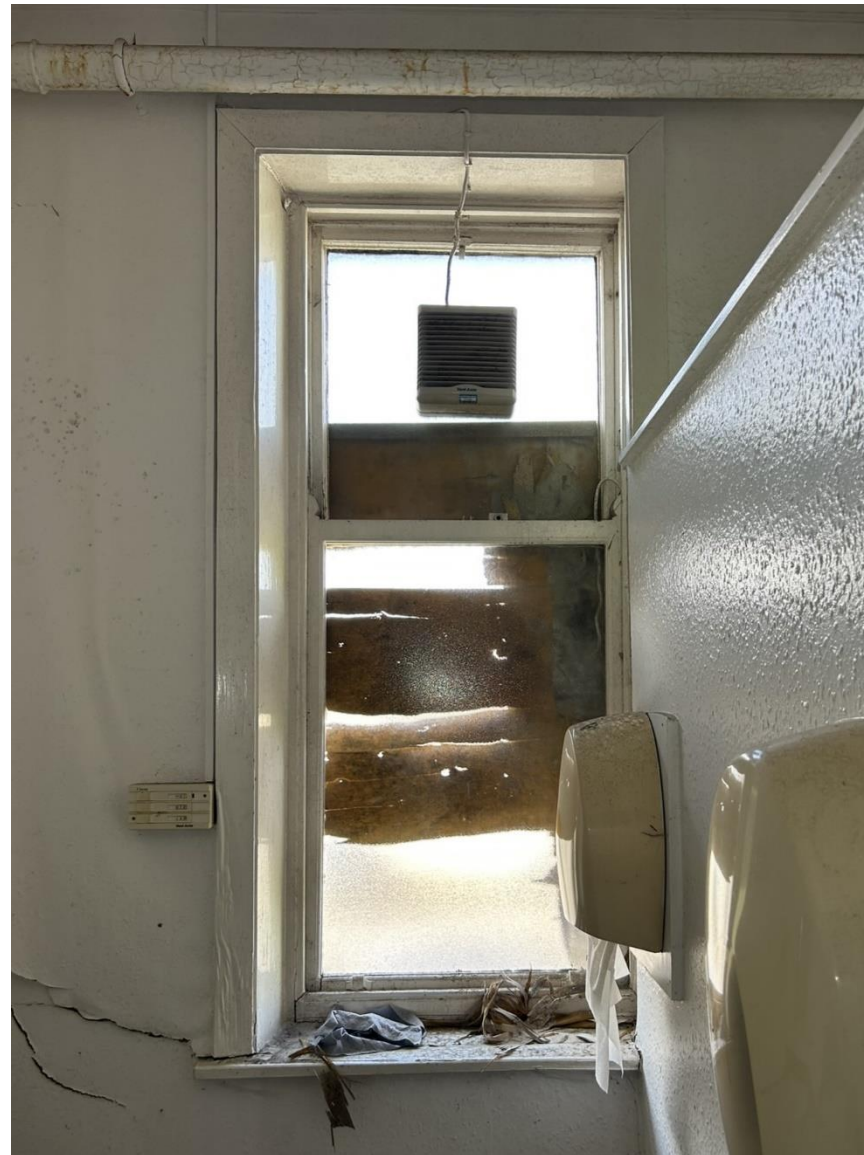
Photo 18.2: Modern & crude joinery to window
