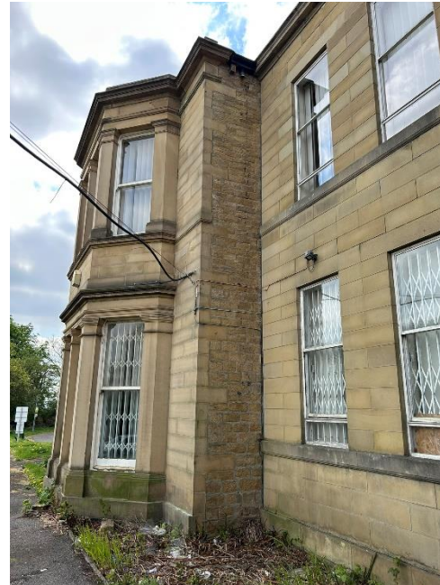
Photo C: Close-up of join between Acre House & link extension to front, which shows that the north elevation of Acre House is/ was faced with random coursed stone
