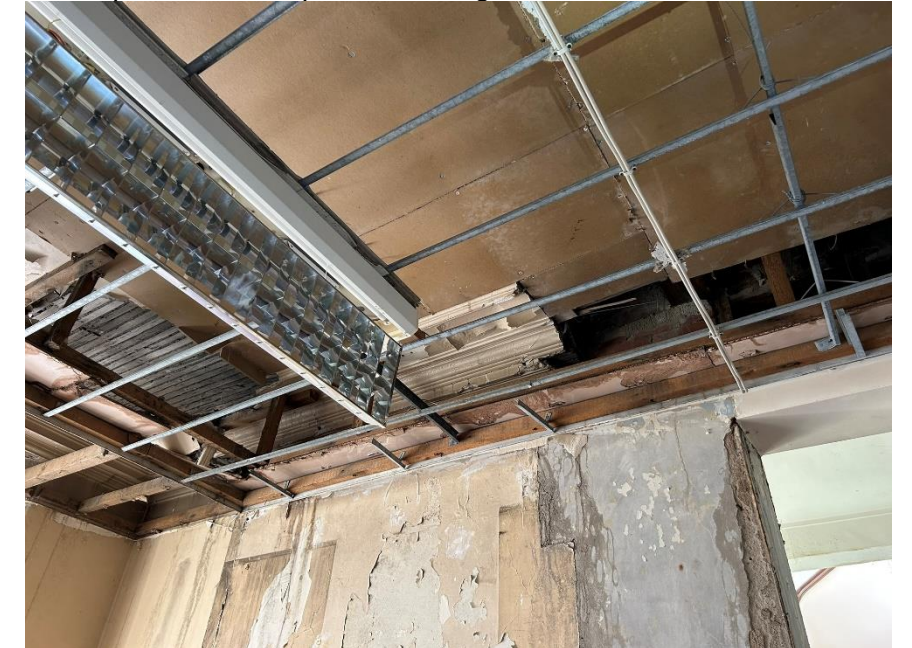
Photo 9.5: Damaged & missing section of cornice to be concealed with replacement suspended ceiling
