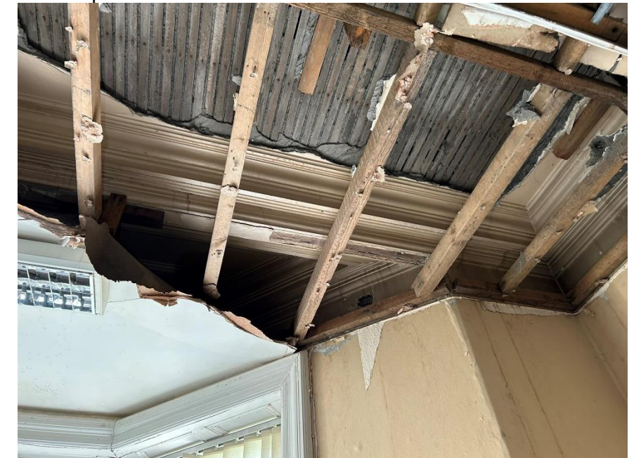
Photo 9.4: Section of surviving cornice over cantered bay window to be exposed
