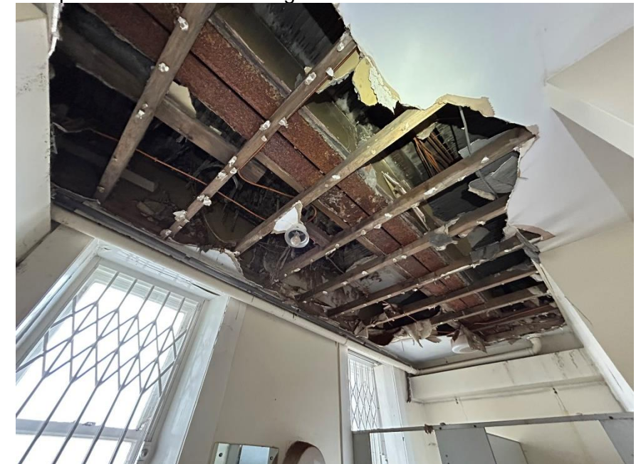
Photo 8.4: Modern plasterboard suspended ceiling, largely collapsed due to water damage
