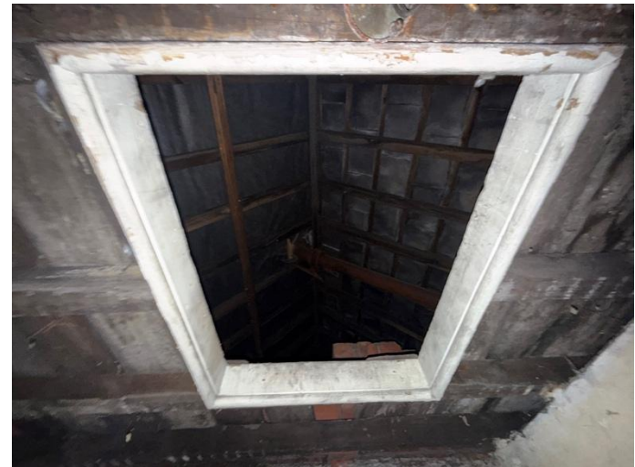
Enclosed void present within northern section of B1
