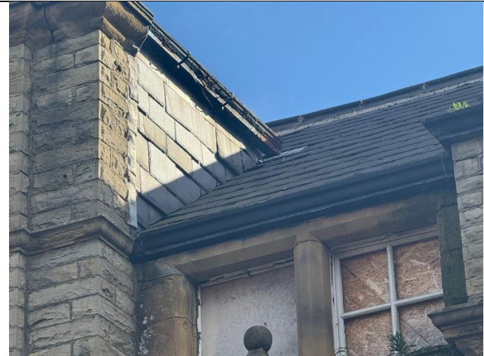
Gaps present around vertical tiles on northern elevation of B1
