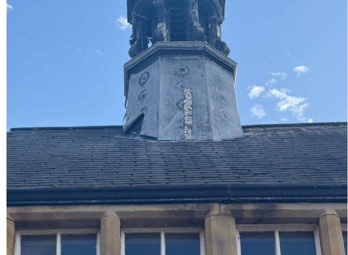
Gaps present around base of tower structure on northern elevation of B1
