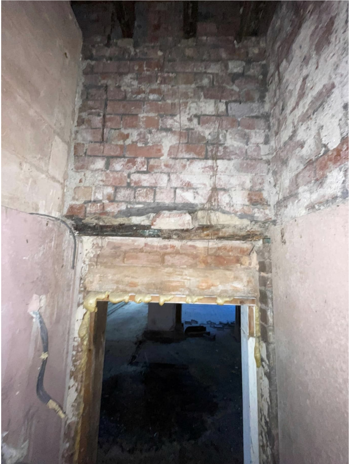
Rotten timber lintel over door opening into small store near toilets.
