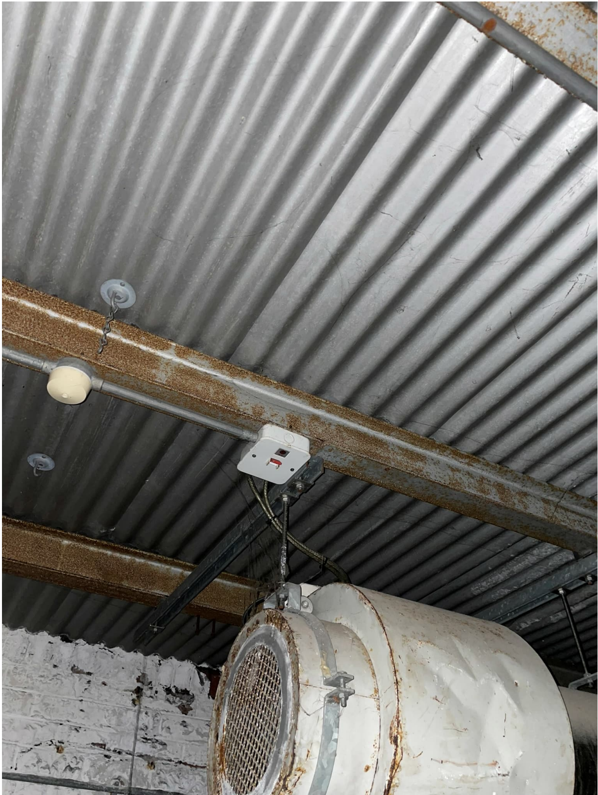
Corroded steelwork grillage in plant/extractor room.
