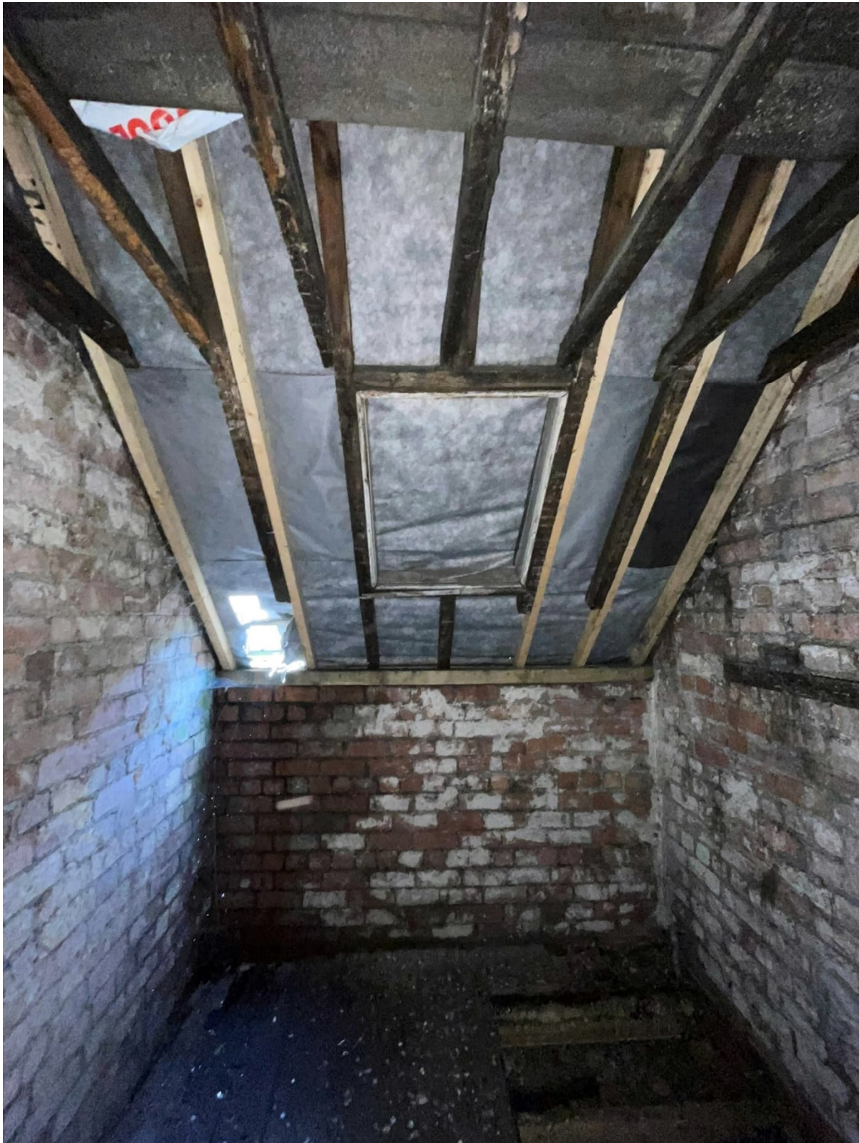
Rotten rafters over front of the building (over entrance).
