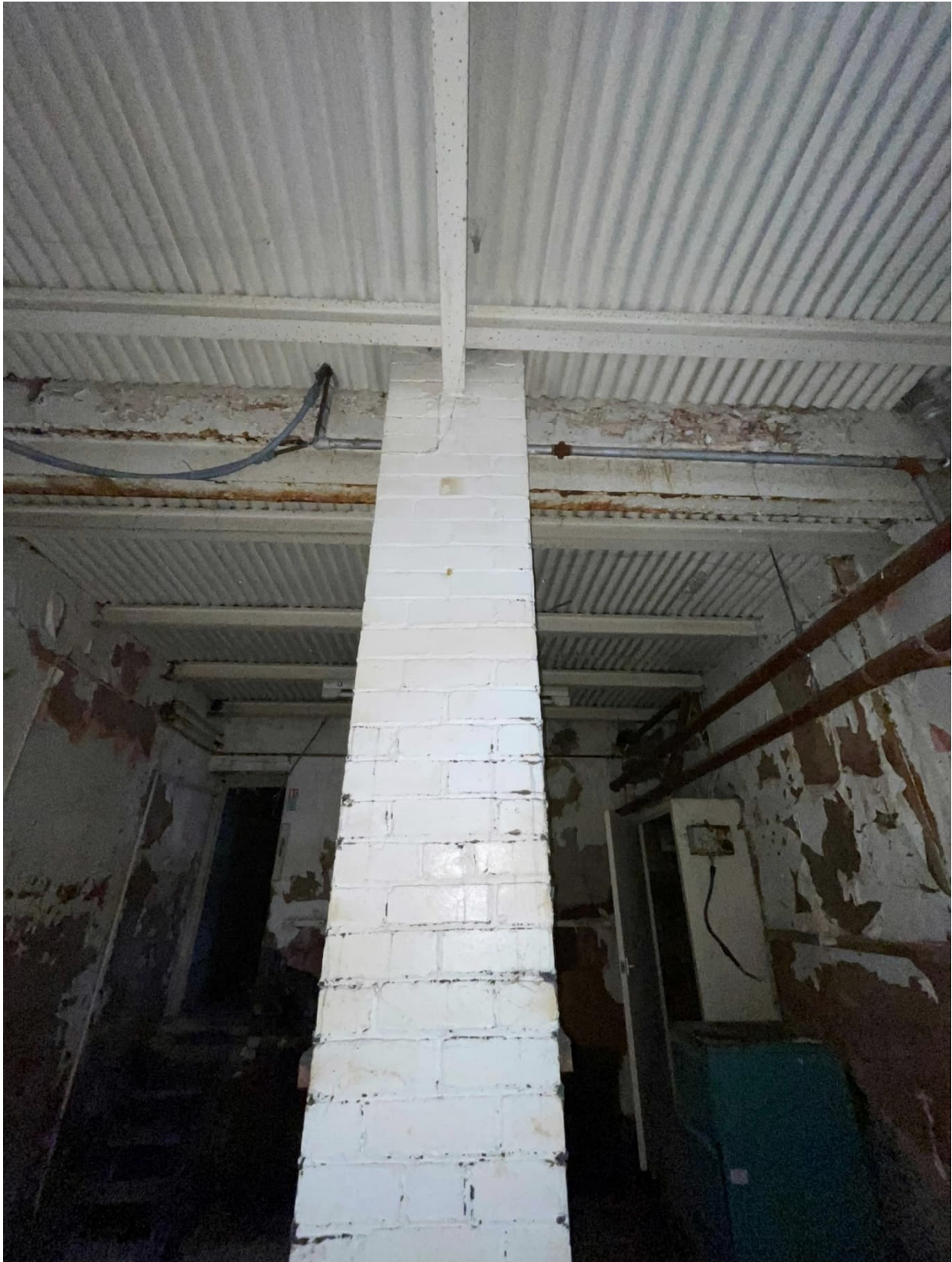
Masonry column supporting steelwork which in turn supports the suspended ground floor.
