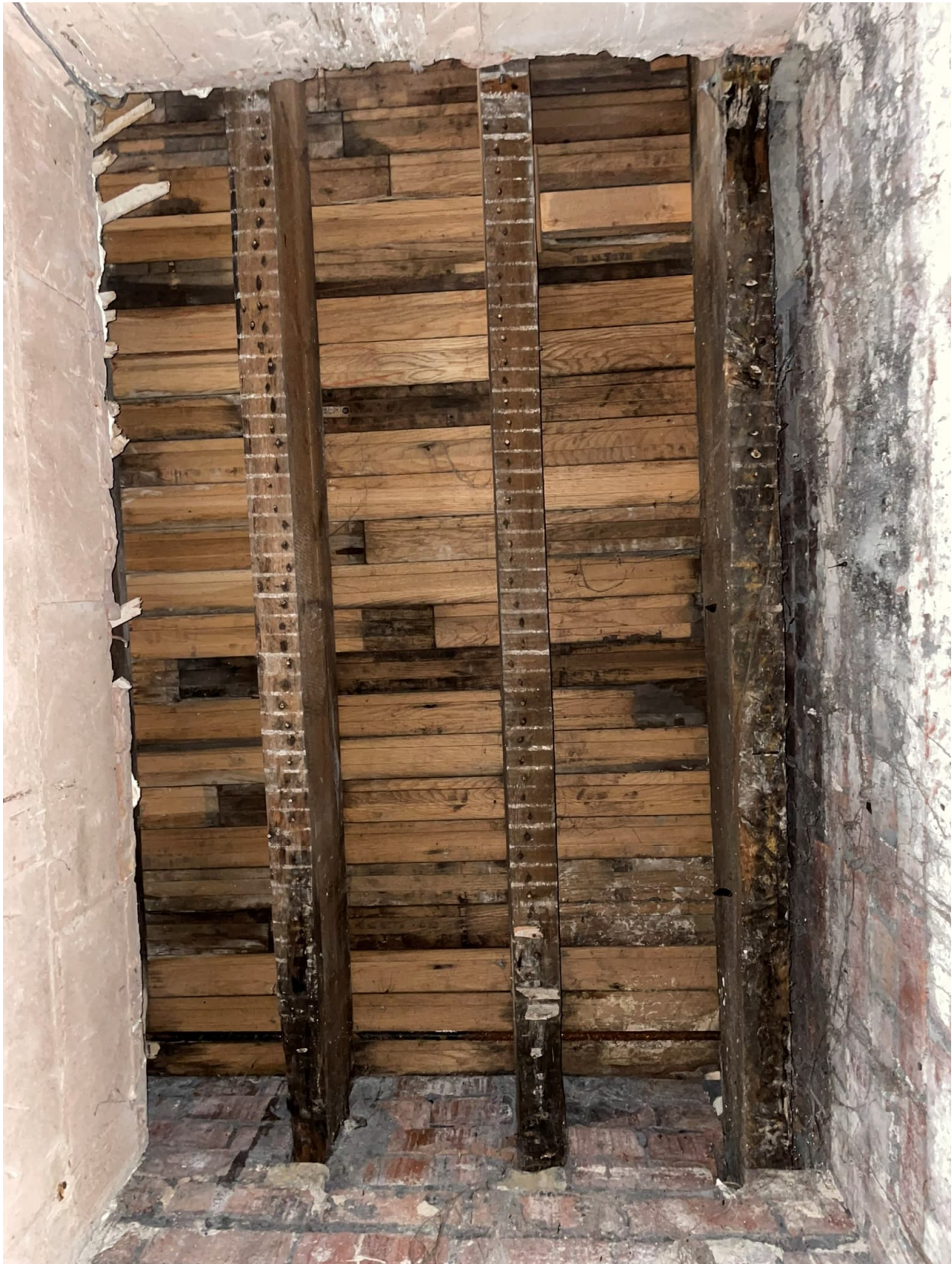
Rotten perimeter joists and rotten joist ends to first floor joists over toilets/store area.
