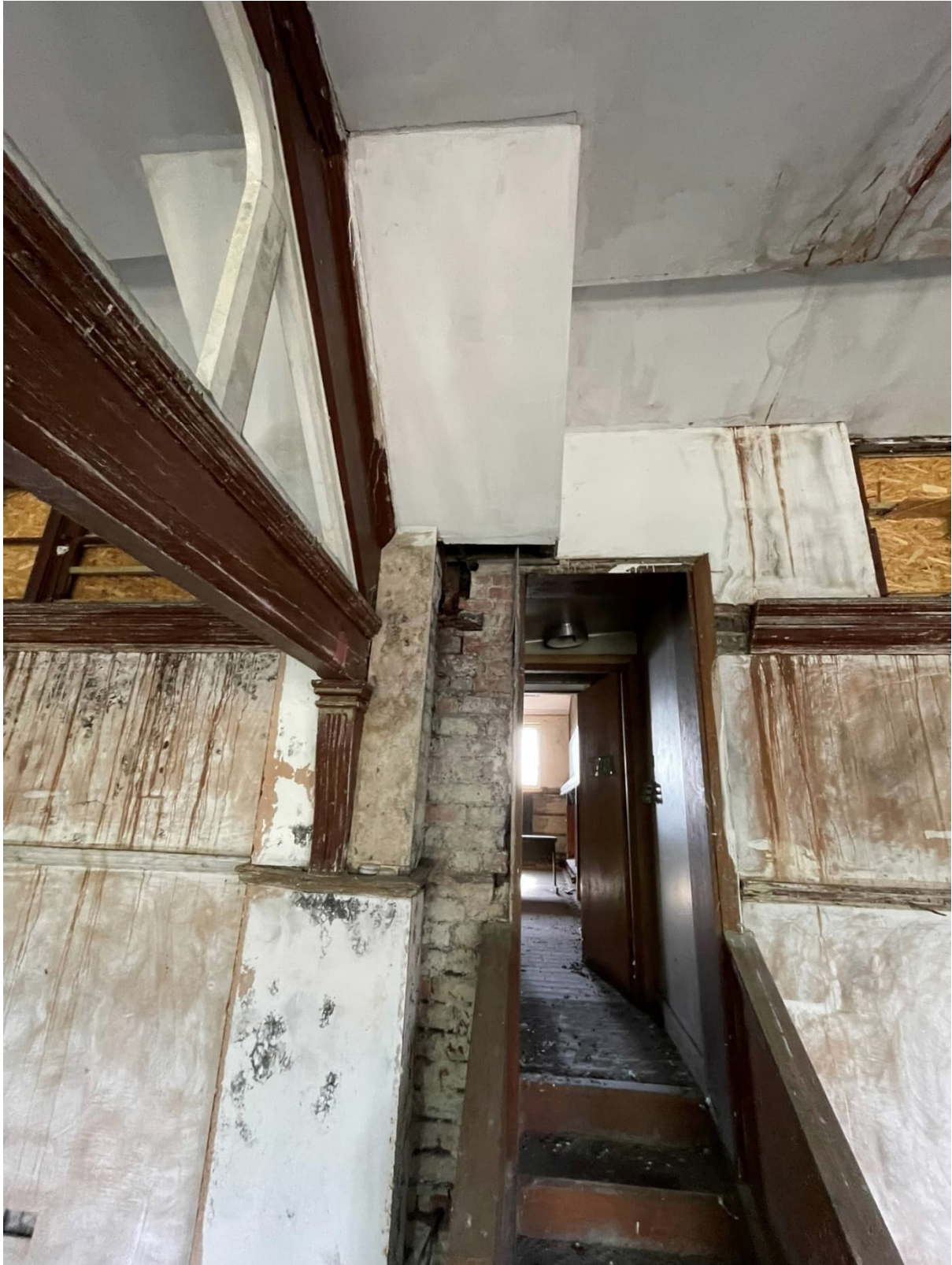
Poor quality masonry to masonry pier supporting truss.
