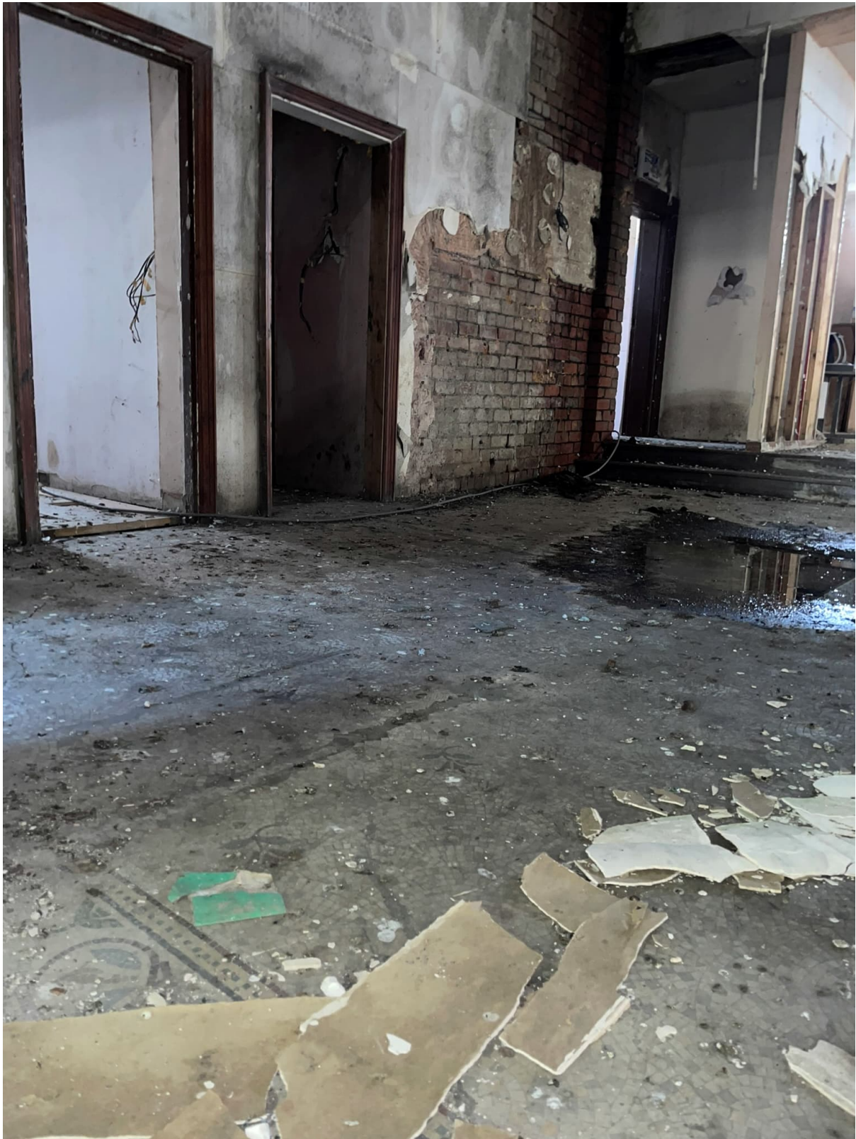
Sunk/bowing ground floor where water is pooling.
