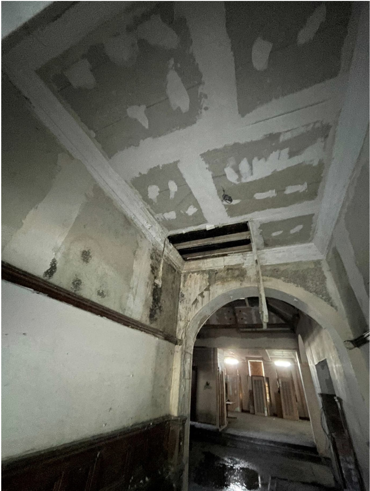
Signs of damp in entrance hallway.
