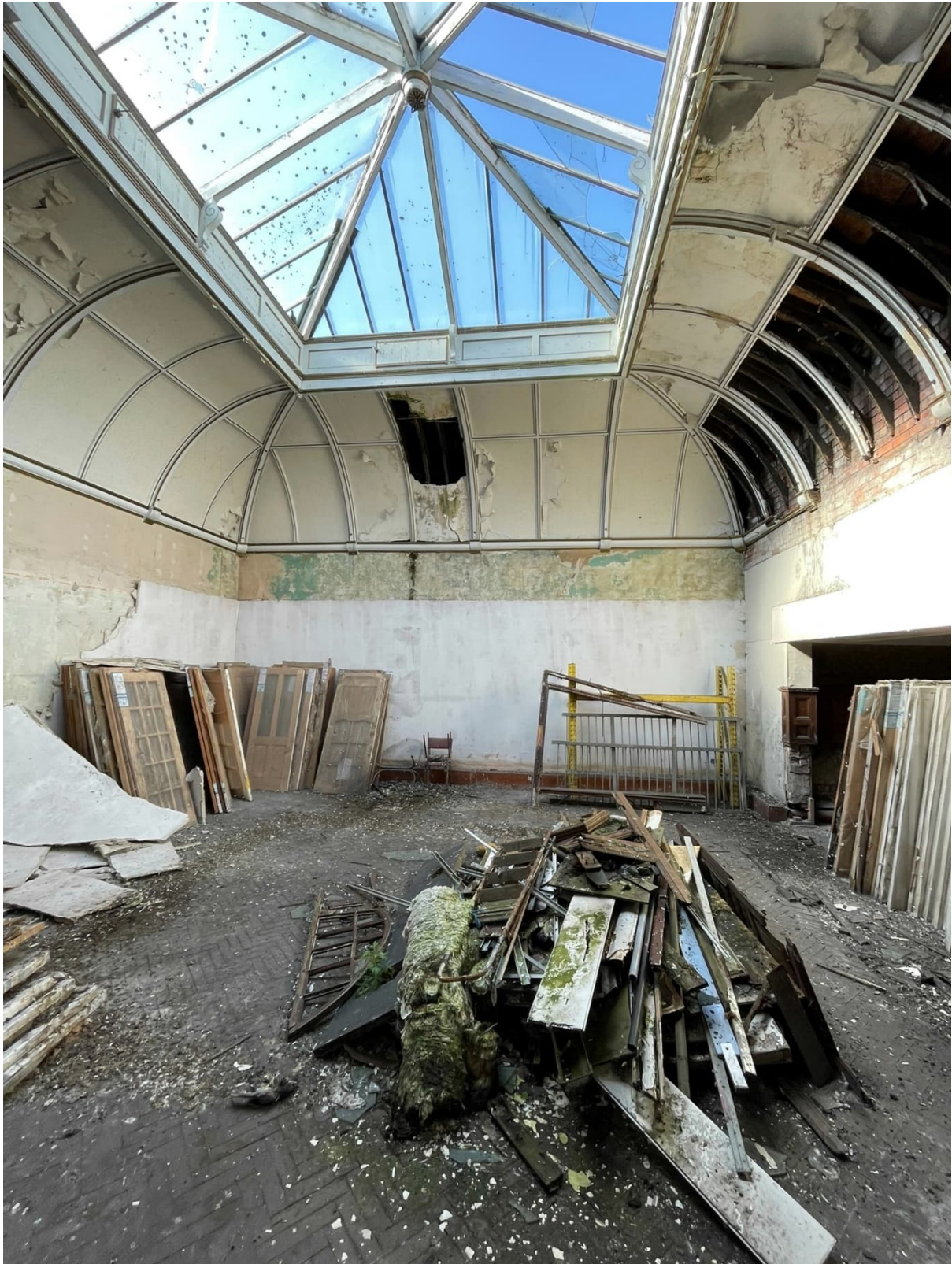
Large damaged lantern and rotten rafters where they bear onto brickwork.
