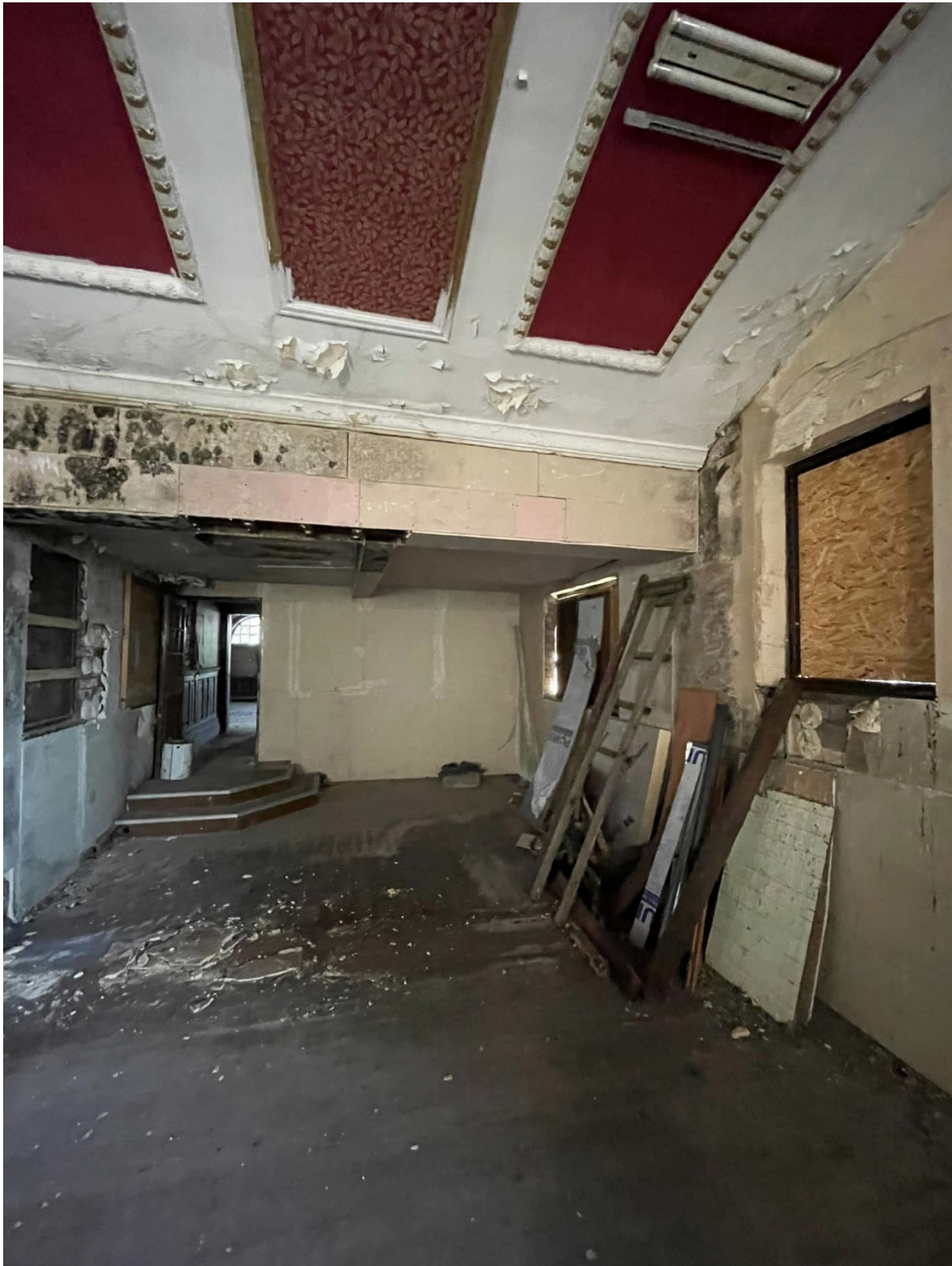
Downstand beams and damp over north-east of first floor hall.
