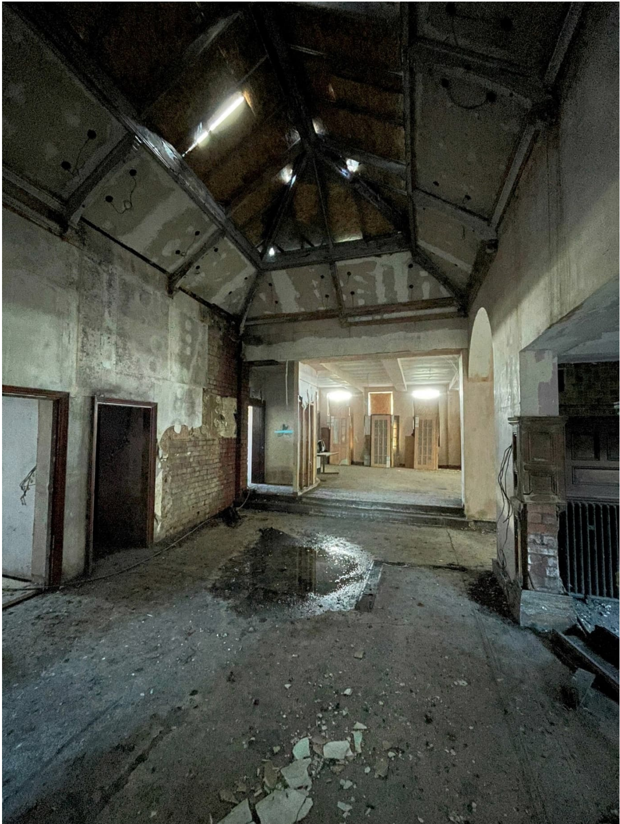
Boarded up lantern & water pooling on the ground floor.
