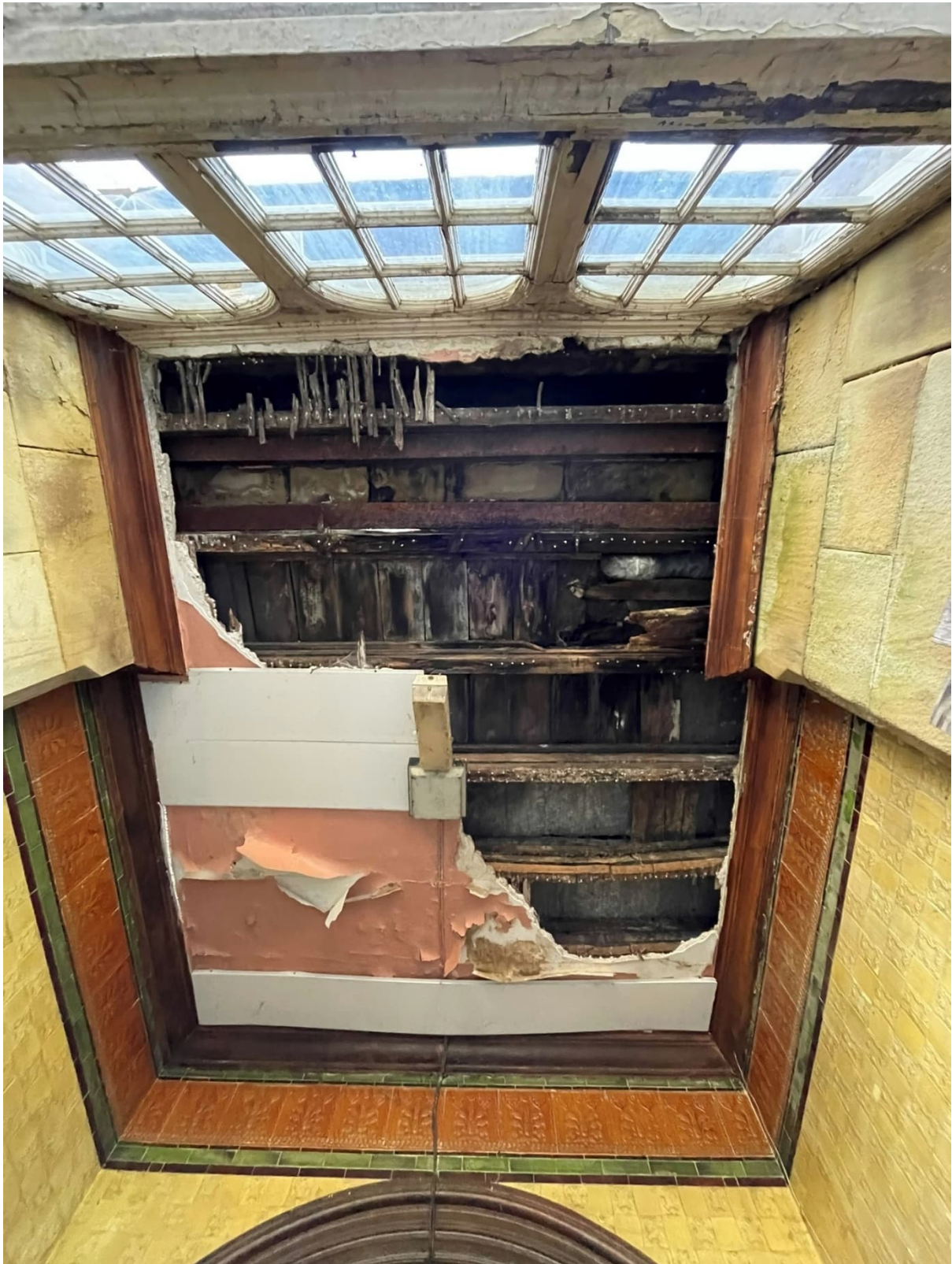
Rotten joists and corroded steelwork over entrance.
