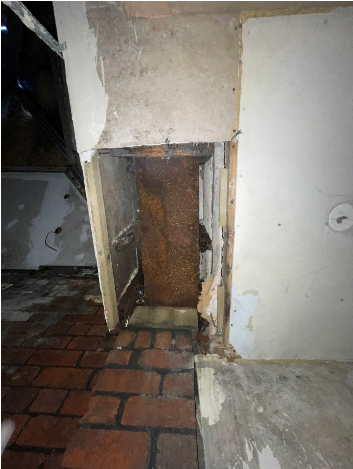
Corroded RSJ with rivets at first floor level.
