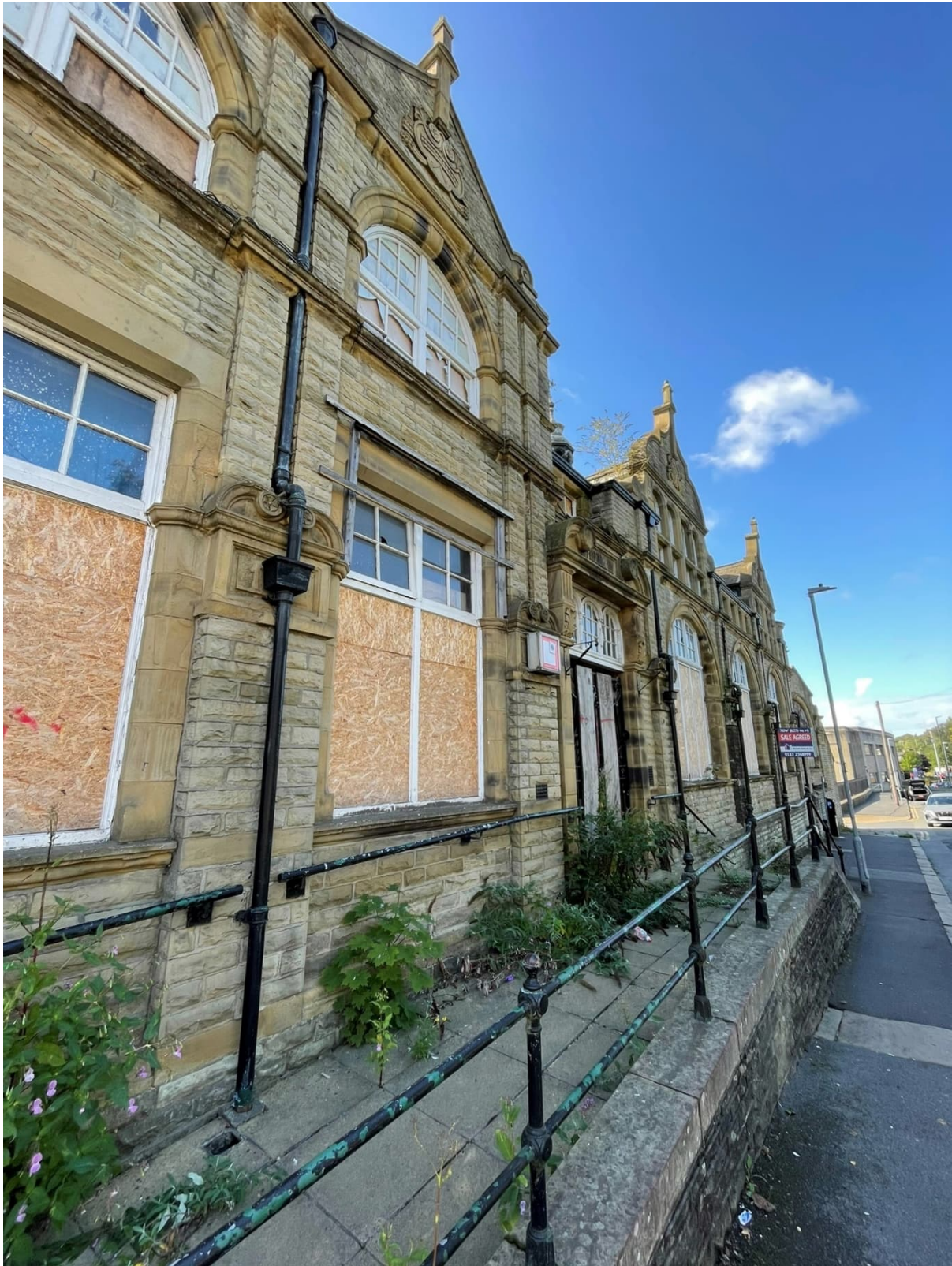
Front elevation, boarded up windows, weathers sills and missing mortar.
