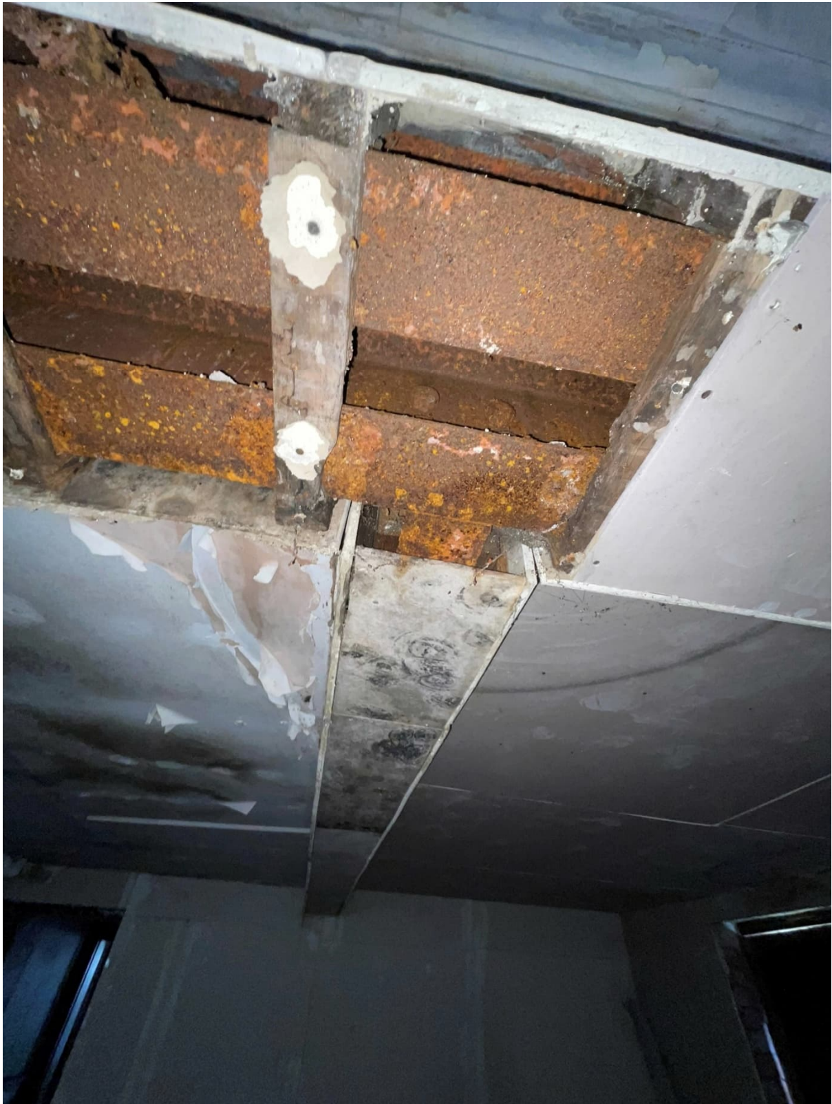
Heavily corroded steel beams over north-east of first floor hall.
