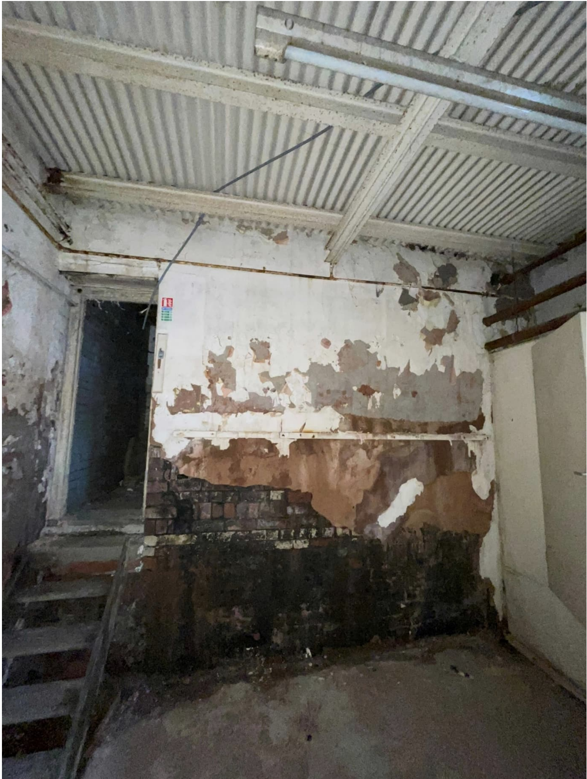
Signs of damp at low level on basement walls.
