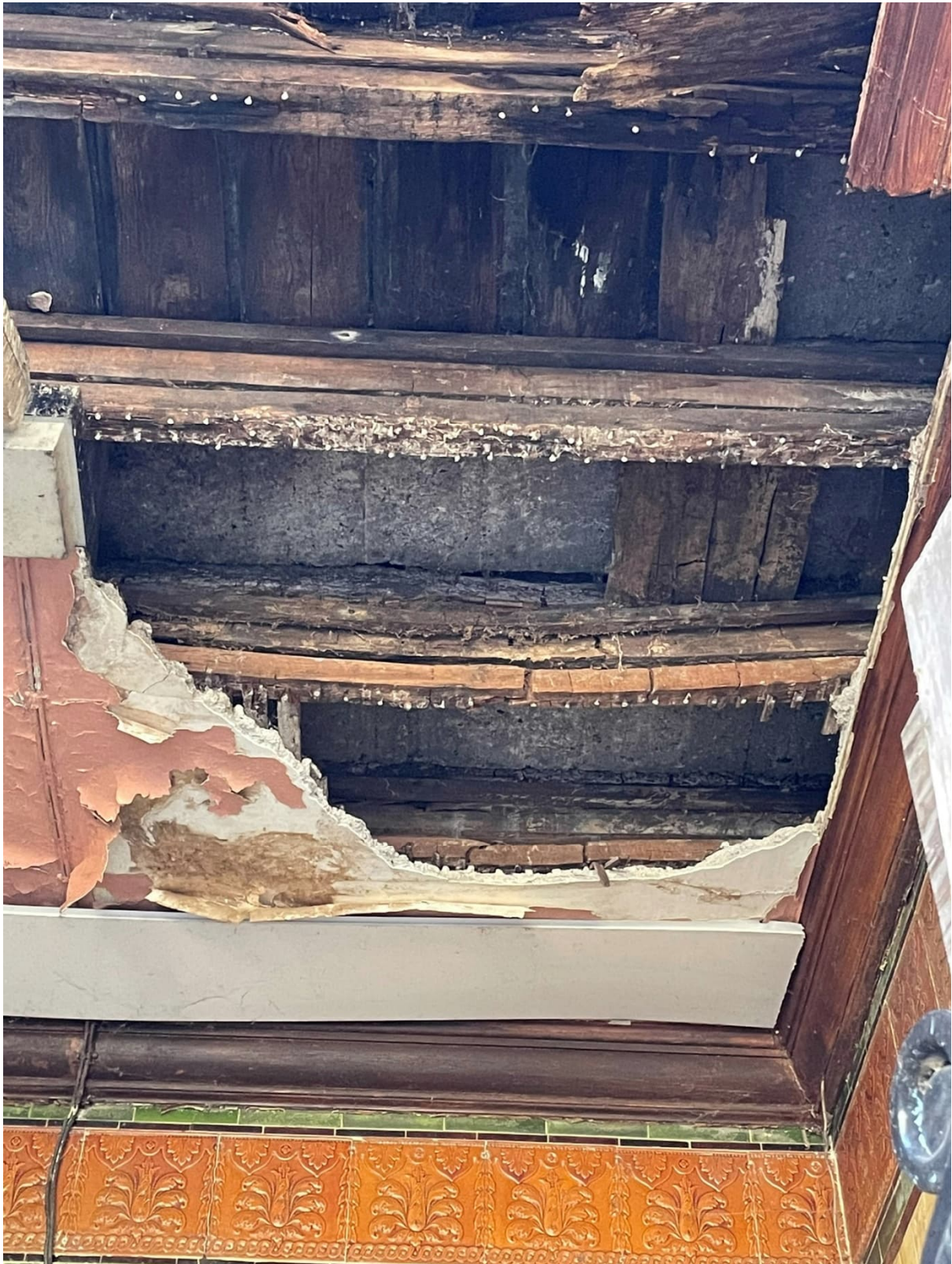
Rotten joists over entrance.
