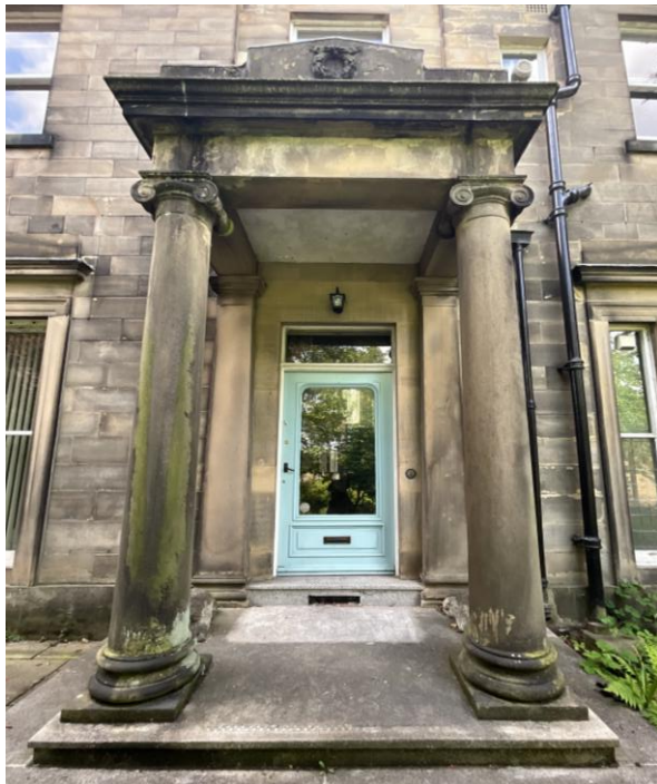
Figure 4: Grade II Listed Entrance Columns. View of the classical stone entrance portico, including the original columns which are Grade II listed. These features will remain entirely unaffected by the proposed change of use.
