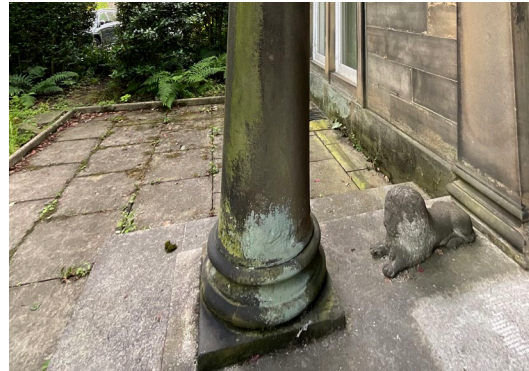
Figure 6: Close-up of Grade II Listed Left Lion Statue. Detail of decorative stone lion located at the left side of the main entrance, forming part of the Grade II listed entrance features. This element will remain untouched.
