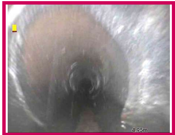
2, 00:00:13, 4.95 m Fracture, circumferential from 7 o'clock to 5 o'clock
