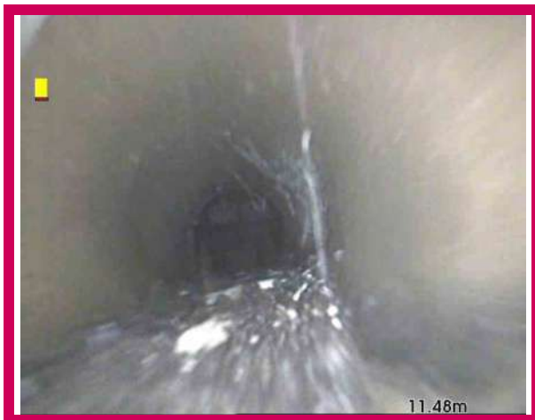
3, 00:00:24, 11.48 m Settled deposits, fine, 15% cross-sectional area loss
