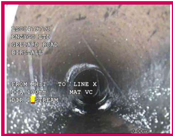
1, 00:00:00, 0.00 m Start node, manhole, reference: MHS1
