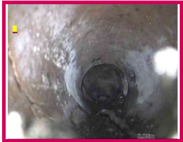
2, 00:00:04, 0.08 m Fracture, circumferential from 7 o'clock to 10 o'clock
