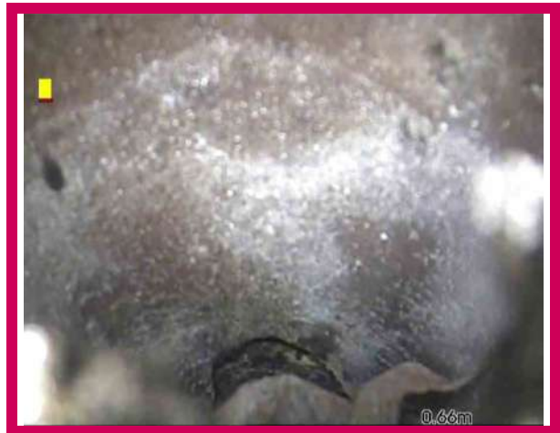
4, 00:00:10, 0.66 m Survey abandoned, Unable to pass debris
