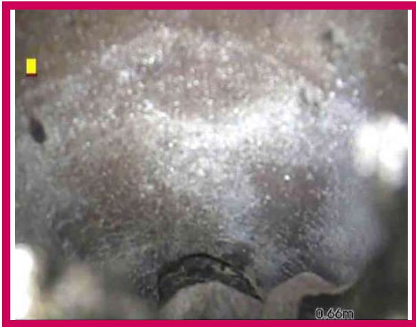
1, 00:00:00, 0.00 m Start node, manhole, reference: MHF1
