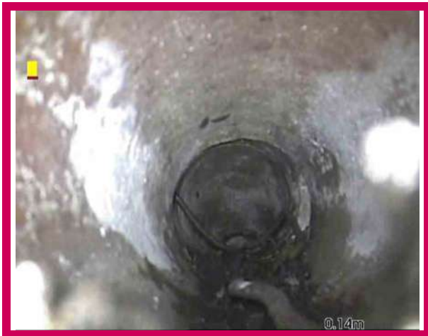
3, 00:00:05, 0.14 m Roots, tap at joint
