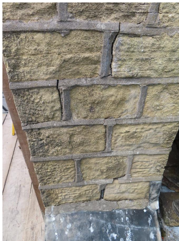
Photo 8 – Cracking was seen on all faces of the chimney stack.
