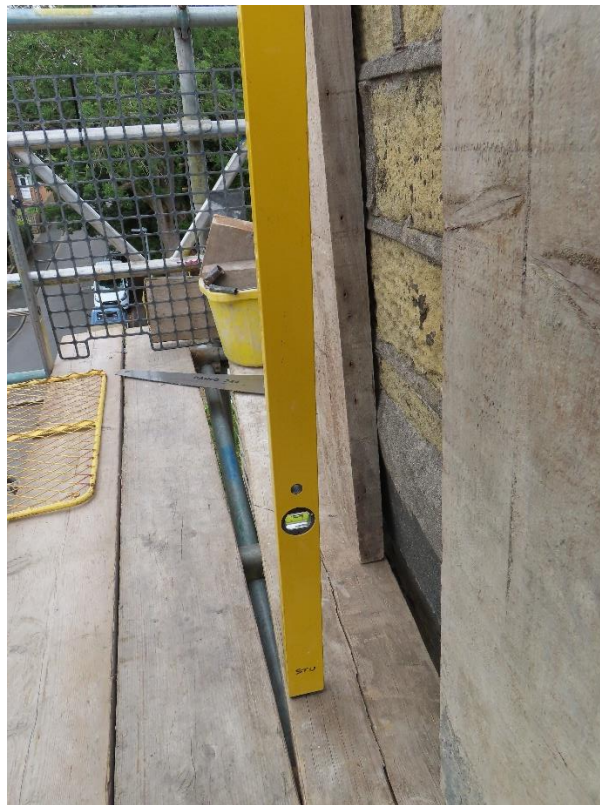
Photo 1 – Chimney lean at the top measured as 200mm out of plumb.
