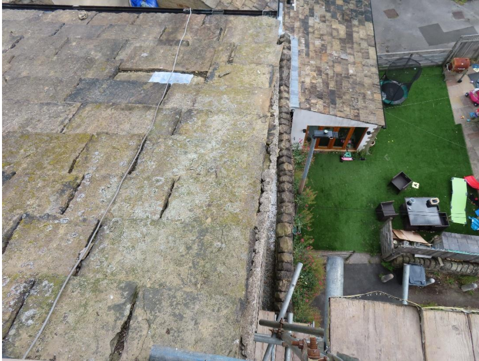
Photo 5 – Exposed top of the stone leaf can be seen as the external leaf of the gable walling has moved out. The stone roof 'slate' finishes are fixed to roof rafters, which are fixed to purlins sat on the inner leaf. Evidence that the inner leaf is moving out far less than the outer leaf stonework.
