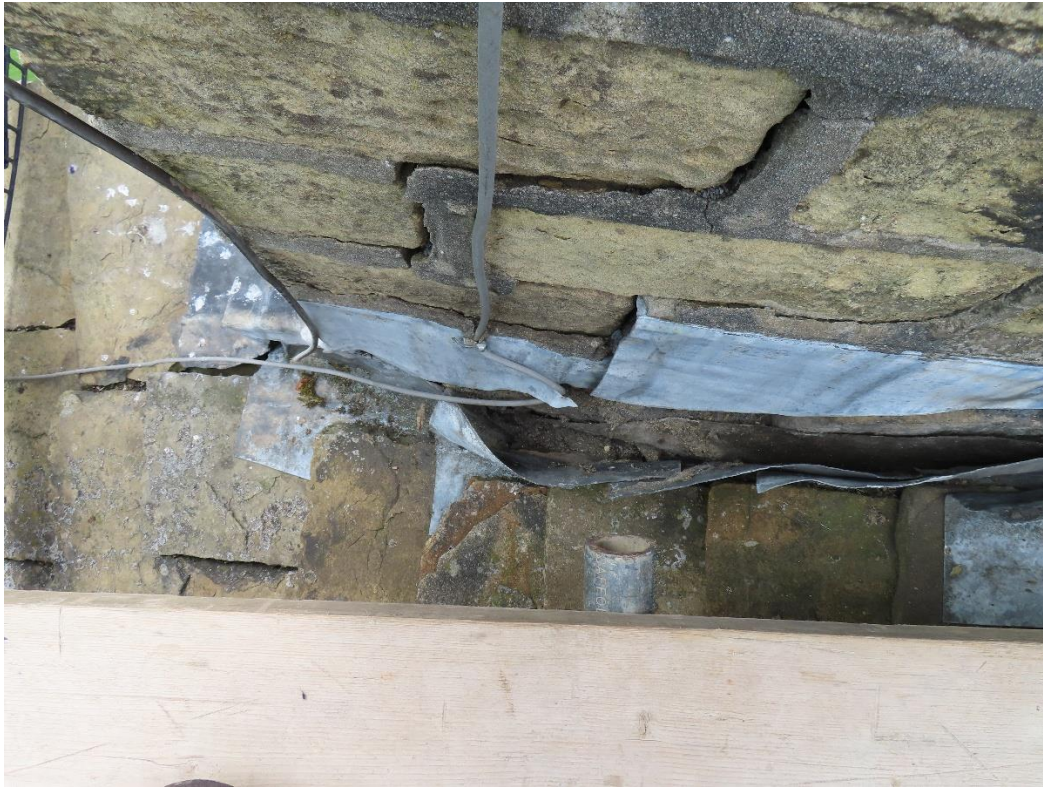
Photo 7 – Massive cracks to the rear of the chimney stack and tearing away of the lead flashings were seen.
