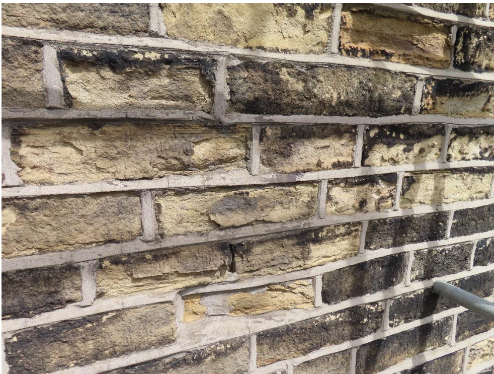
Photo 6 – Dozens of tension cracks were seen to the gable pointing as the gable external leaf moves out, increasing the curvature of the external leaf.
