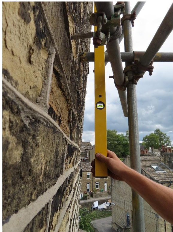
Photo 3 – Top gable lean from front sill stone level upwards. Lean at the front of the gable was measured as 90mm approx. to this 1.35m height above the sill stone level.
