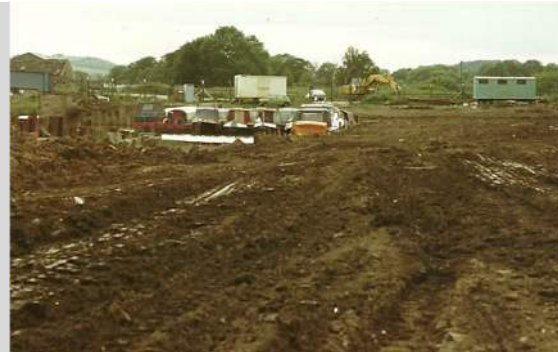
12. Arisings used to infill drainage ditch and lagoon to rear of dry dock, after new culvert installed
