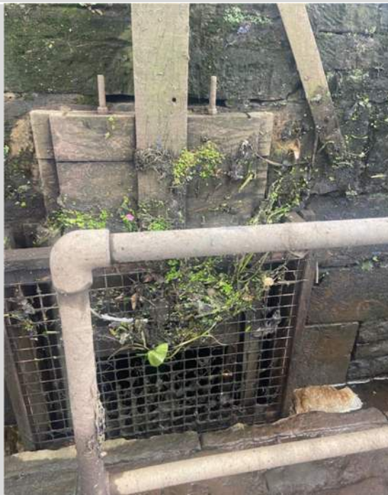
11. Sluice gate at northeast end of dry dock. The drainage ditch and lagoon have been replaced with a culvert that feeds directly into the River Calder.
