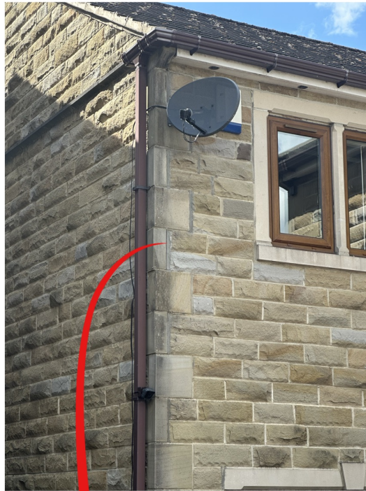
Images 4-5: Evidence of foundational movement in original stonework at the corner of my home
