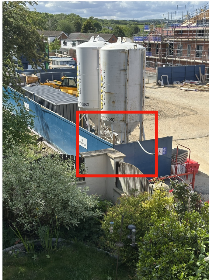
Images 8-9: Photographs showing the proximity of the proposed substation to my rear garden boundary from west-facing bedrooms
