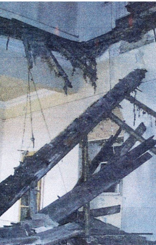
Photo from structural report, Gifford & P., 2000. Dining Room - first floor collapsed.
