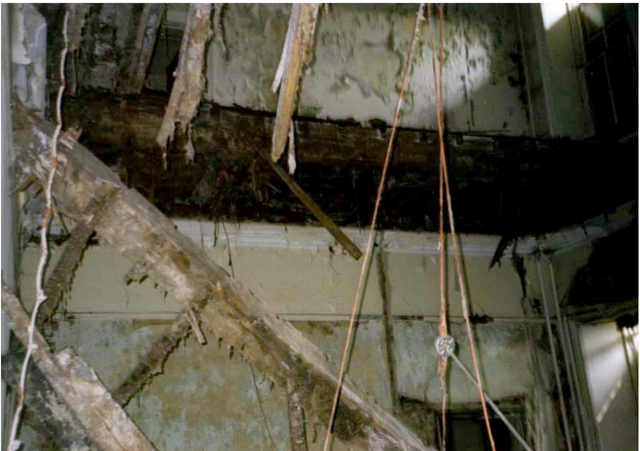
Archive photo of the interior of The Mansion House at Storthes Hall (pre 2000) showing collapsed flooring.
