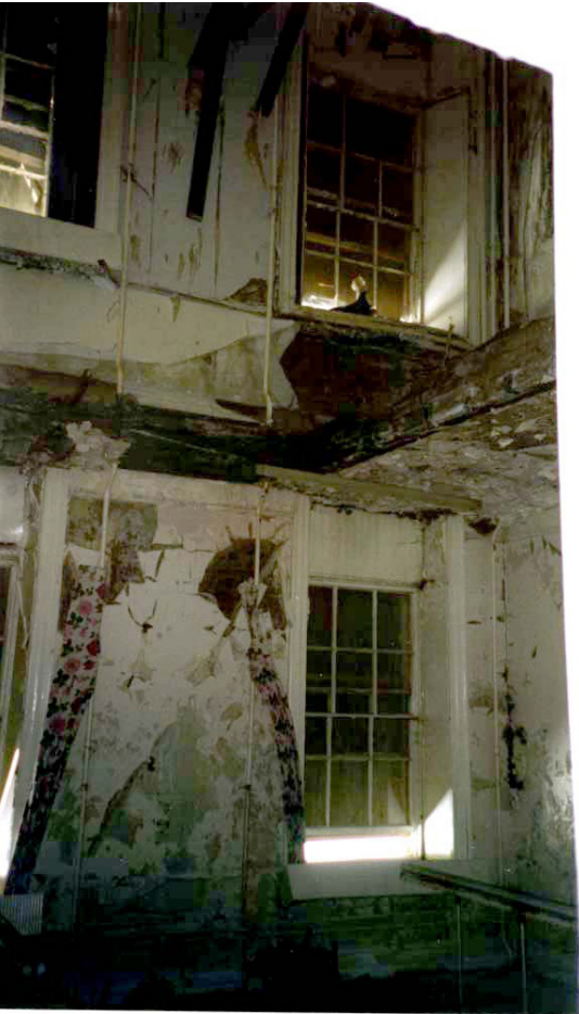
Archive photo of the interior of The Mansion House at Storthes Hall showing collapsed flooring (pre 2000).
