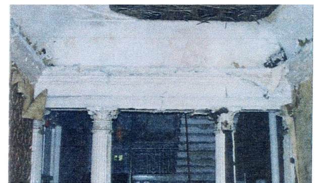
Photo from structural report, Gifford & P., 2000 Entrance Hall - plaster to ceiling and timber columns damaged, beam cracked.
