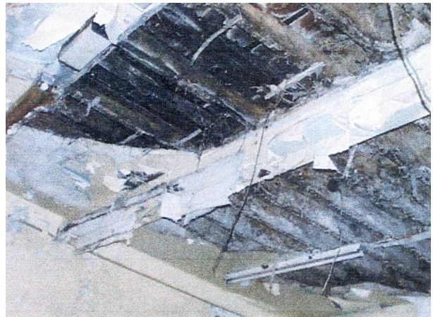
Photo from structural report, Gifford & P., 2000 Boot room - plaster fall to ceiling and decay to timber.
