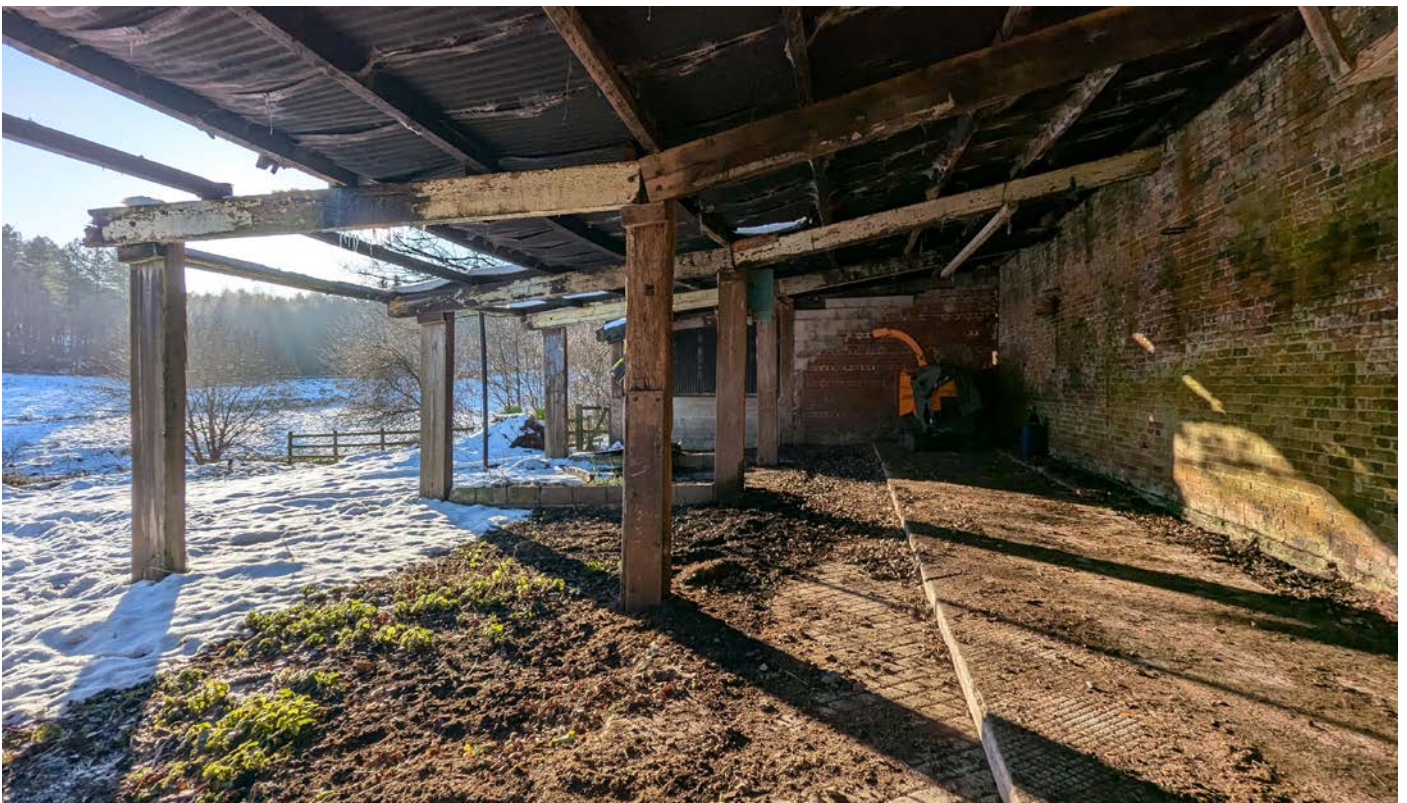
Existing store, looking west - there is some subsidence to the central columns where no concrete slab is present.
