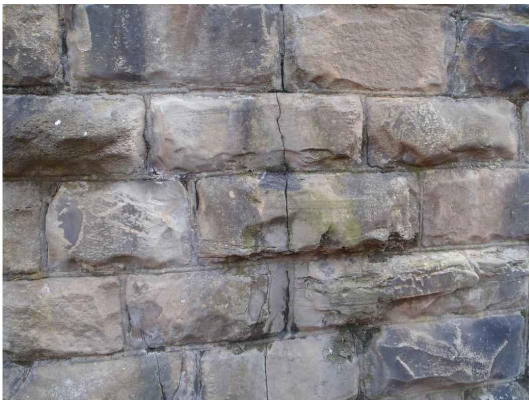
Insert 1-3 Example of a longitudinal fracture within the masonry of the viaduct.
