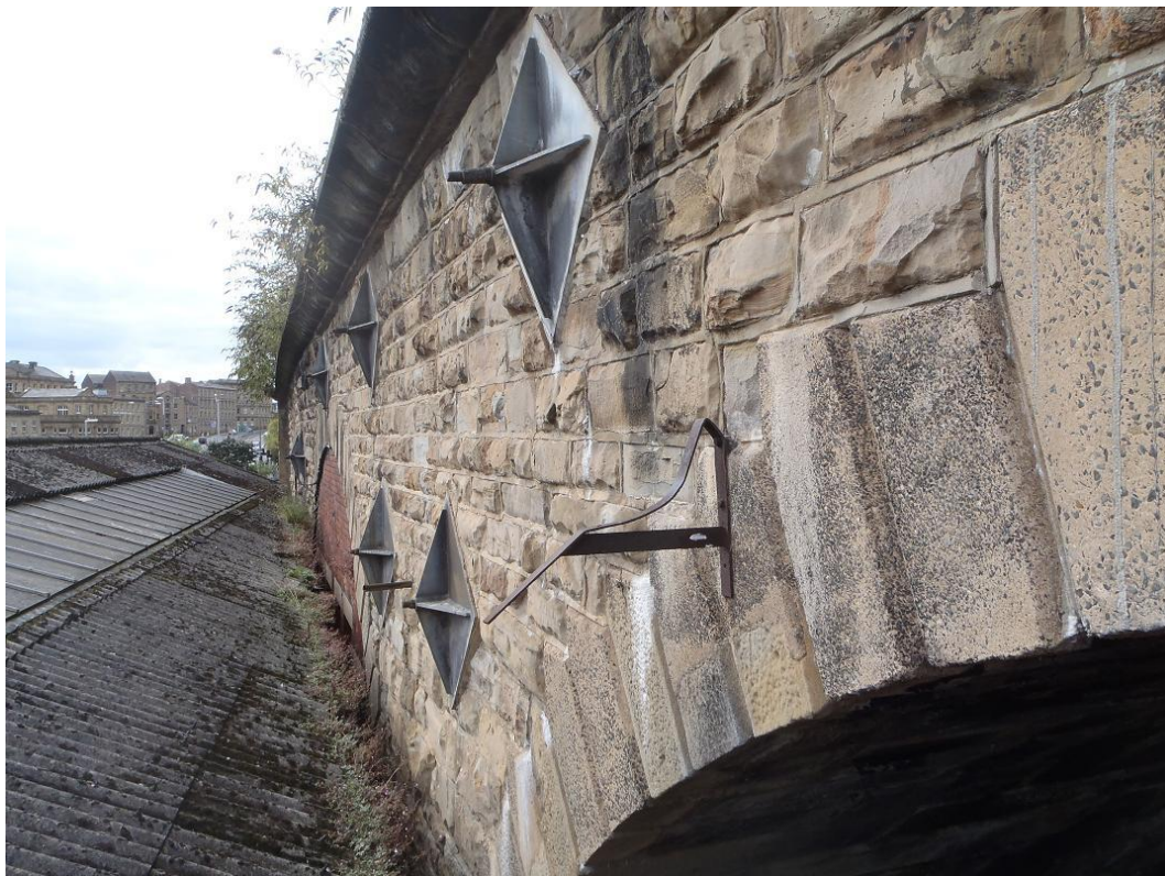
Insert 2-7 Proximity of buildings to Spans 8,9 and 10 and pattress plates (eastern elevation).
