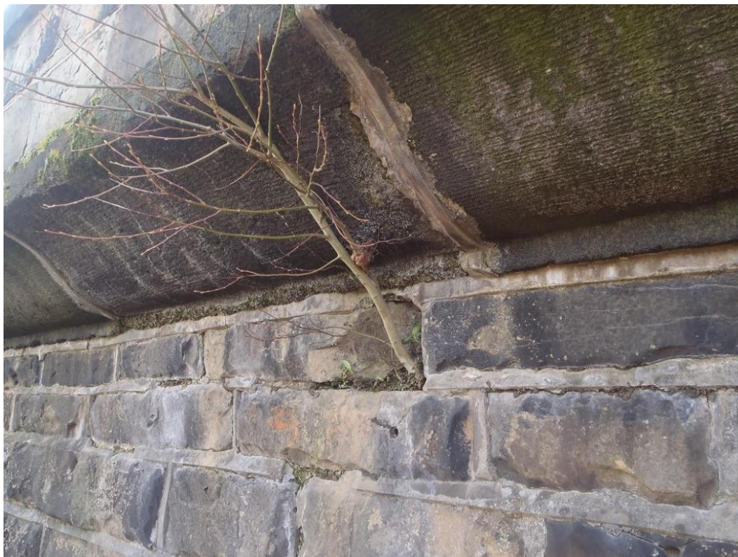
Insert 1-2 Evidence of spalling and vegetation growth.
