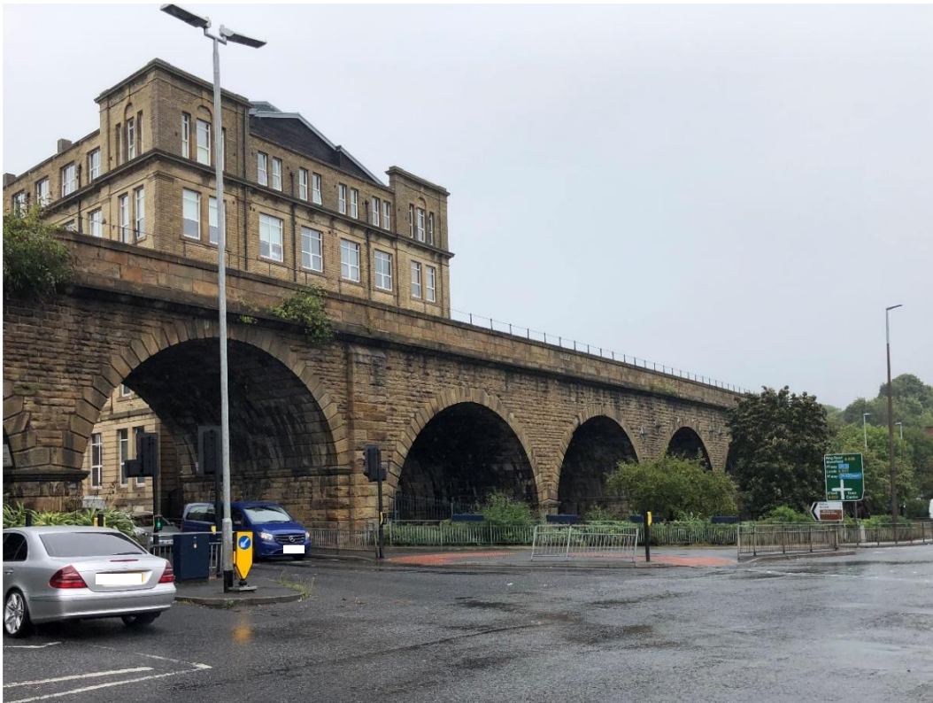
Insert 1-1 Dewsbury Viaduct (MDL1/19) from south-east, showing Spans 3 to 6, with former Spinkwell Mill in the background.
