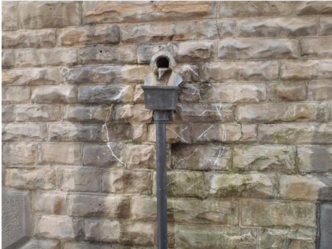
Insert 1-4 Evidence of drainage issues around a downpipe hopper head, with associated dampness and spalling.
