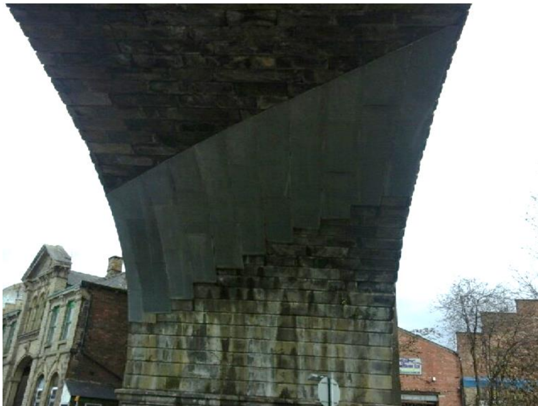
Insert 2-10 Soffit of Span 7, showing later addition of strike protection cladding plates.
