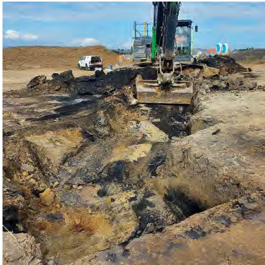
Photograph 04: Coal removal in gardens of Plot numbers 136/137 as per Drawing No. SR3786/VR/P2/05 (20.07.23).
