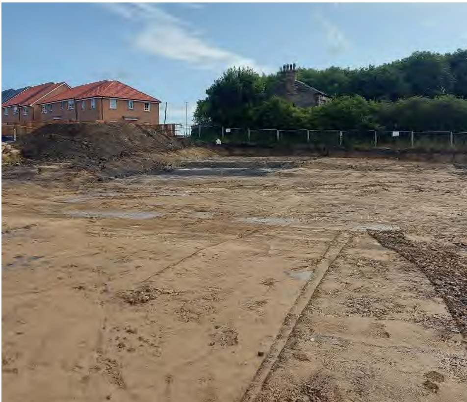
Photograph 09: Cut and fill operations in the northeast of the site and topsoil stockpile (top left) (25.07.23).
