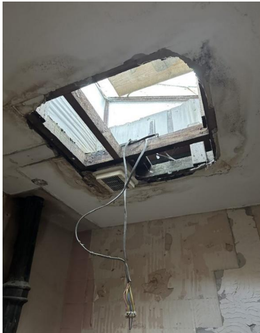
Photo 10. The broken skylight which facilitates bird entry into the building
