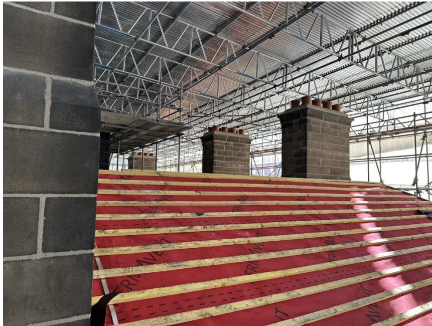
Photo 3. An aspect of the George Hotel roofline running east to west, showing scaffolding
