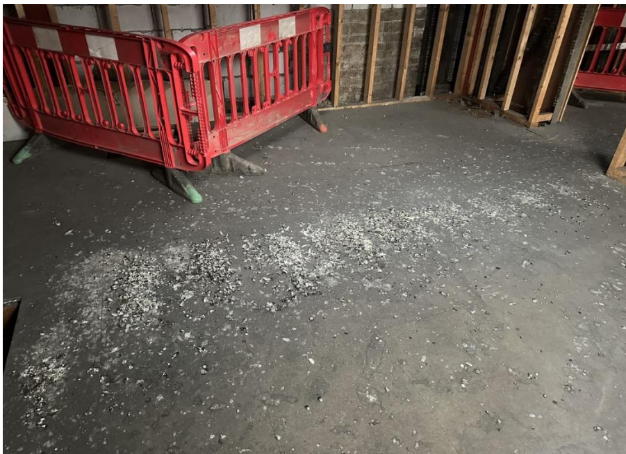
Photo 12. Mounds of pigeon guano in the interior of the building, indicating long-term pigeon presence
