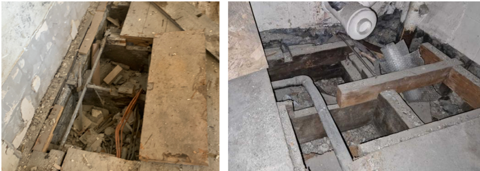
Figure 3 – Heavily Notched Joists (30-40%)
