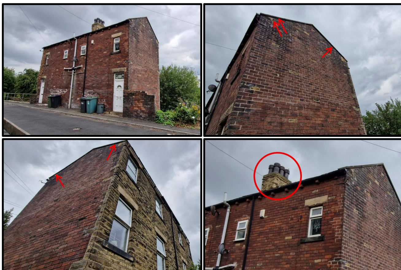
Figure 2: Building with bat roost potential and pigeon nest on chimney.
