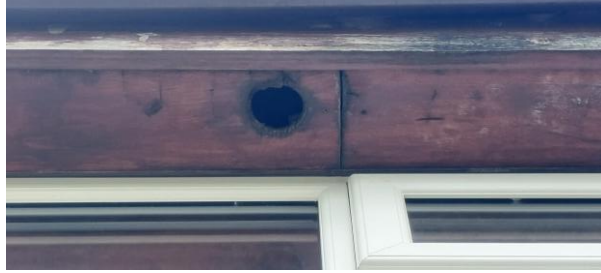
Plate 4: PRF2 missing cover of air vent barge boarding, south elevation.
